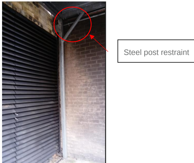
Figure 11 - Steel stair support restraint to Roundhouse Wall.
