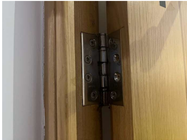
Ensure there are no screws missing in hinges.
