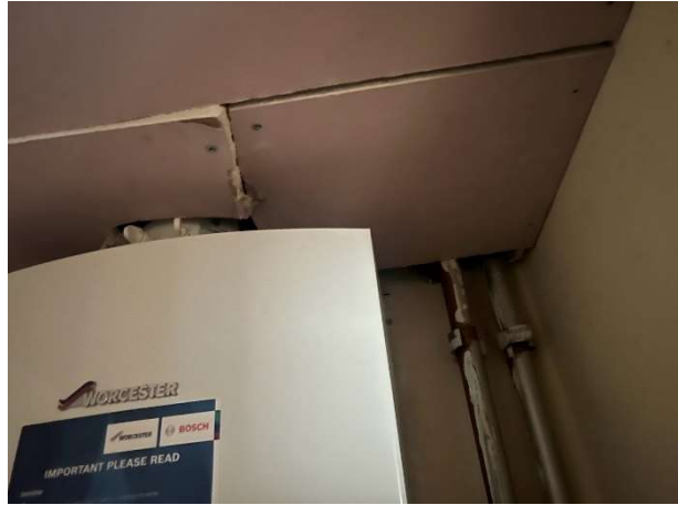
Fire stopping required. Please use mastic not foam.
