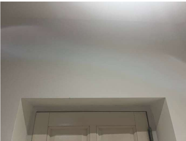
Fire Exit sign required on the main door.
