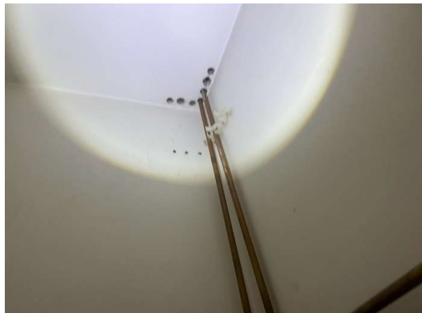
Fire stopping in hole penetration.
