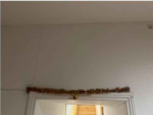
Fire Exit signage in basement required.
