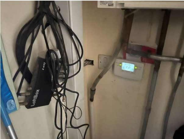
Fire stopping required.
