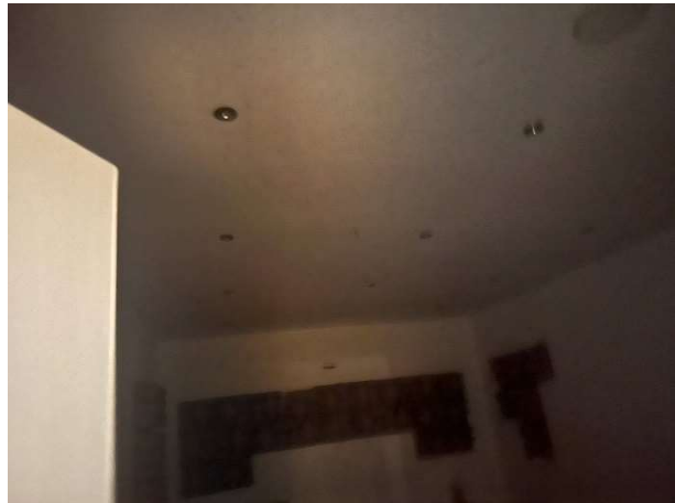
Emergency Lighting Required in common room
