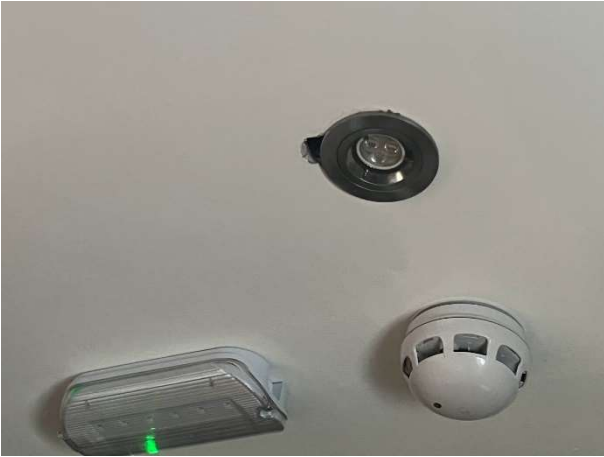
Top floor bedroom – fire stopping around the light.
