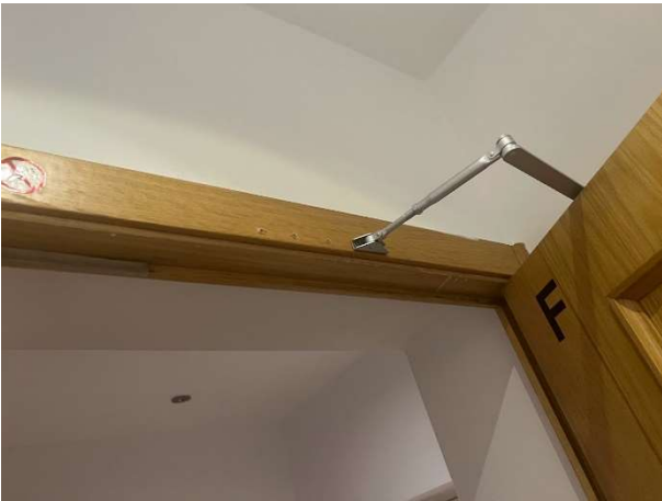
Ensure all doors have intumescent strip with smoke seals.
