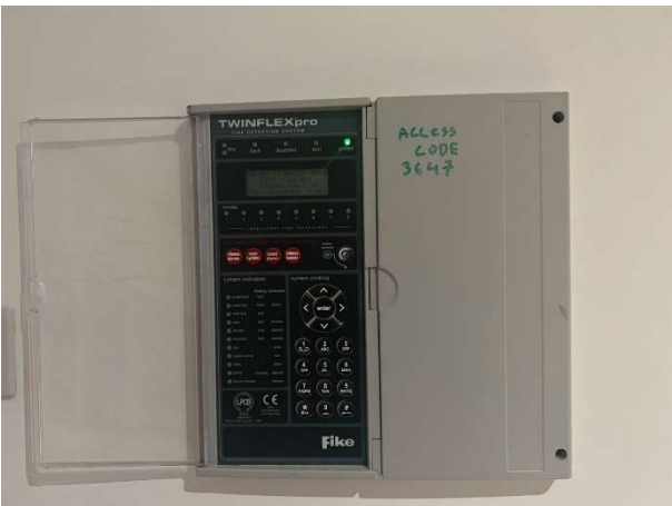
Fire Alarm in good order.
