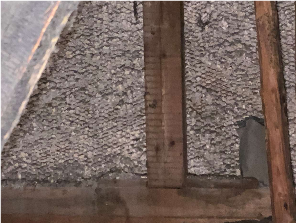
south gable with modern sawn timbers with render on modern metal lath
