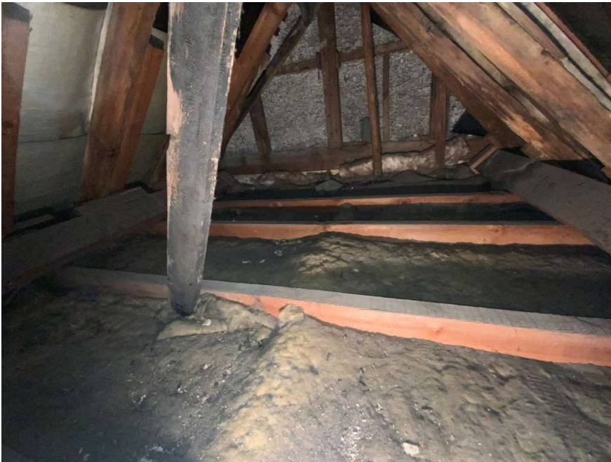
Modern rafters with saw marks and ceiling joists with render on modern metal lath to south gable
