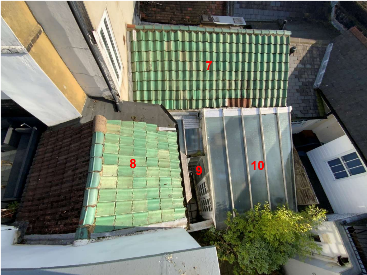
View through showing elements 7,8,9 & 10; note the section of felt roof adjacent to element 8 and the section of glazed monopitched roof over part of element 9 open passageway.
