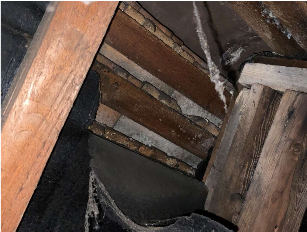
Modern rafters and bituminous felt with modern battens over supporting modern concrete tiles
