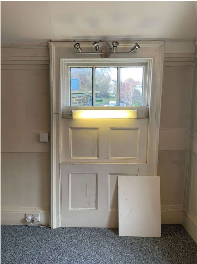
Timber vertical sliding sash window; 3 over 3 configuration; moulded architrave with original 2-part vertical sliding shutters with fixed panelled apron
