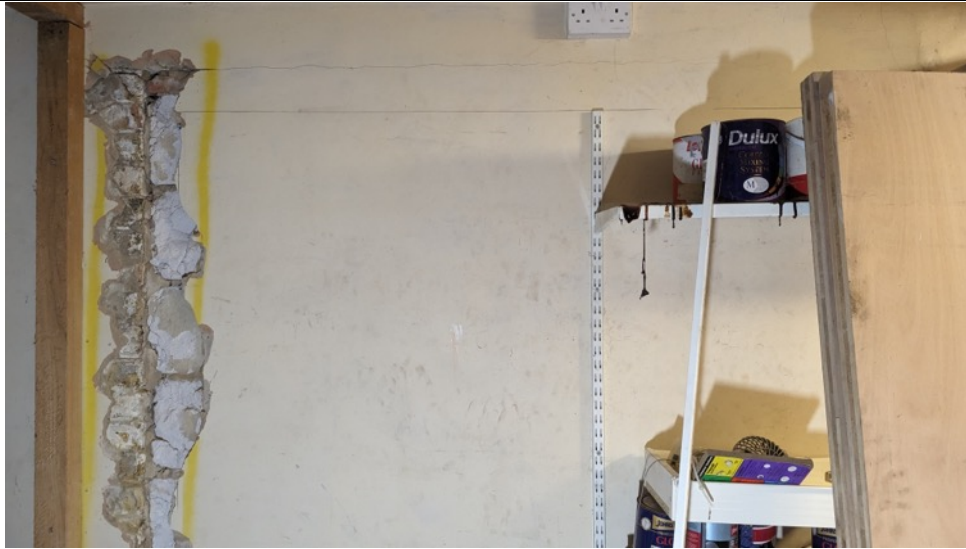
Photo 21: Trial Pit Two adjacent the party wall showing screed, slab, made ground and projecting concrete footing. Depth and extent of concrete footing unknown. Bottom / edge not found
