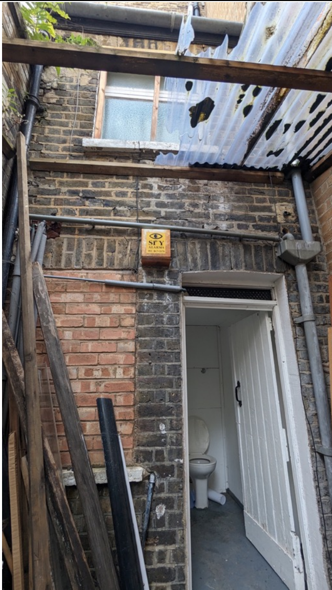
Photo 11: Flat brick arch lintels over door / infilled window have failed. Cracking observed in masonry above
