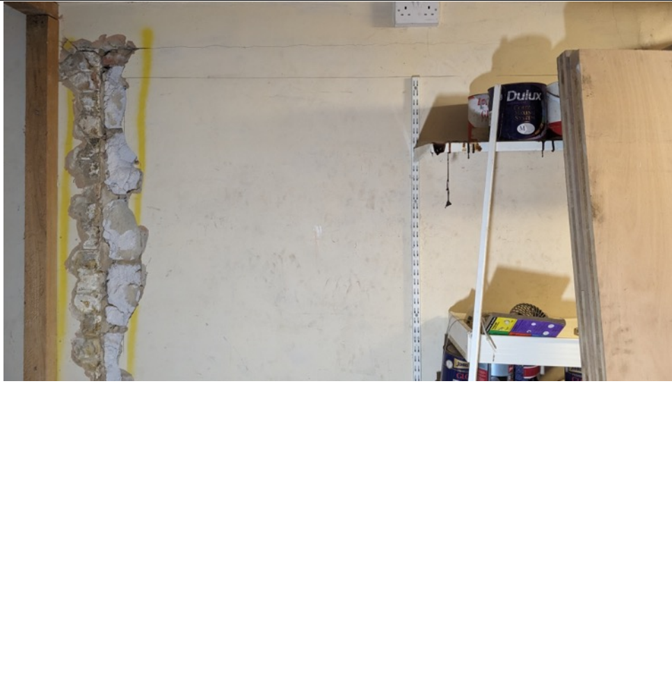
Photo 23: Front wall in basement. Removal of plaster reveals a historic opening has been infilled with blockwork. The cracking of the plaster is superficial and located around the extents of the block infill
