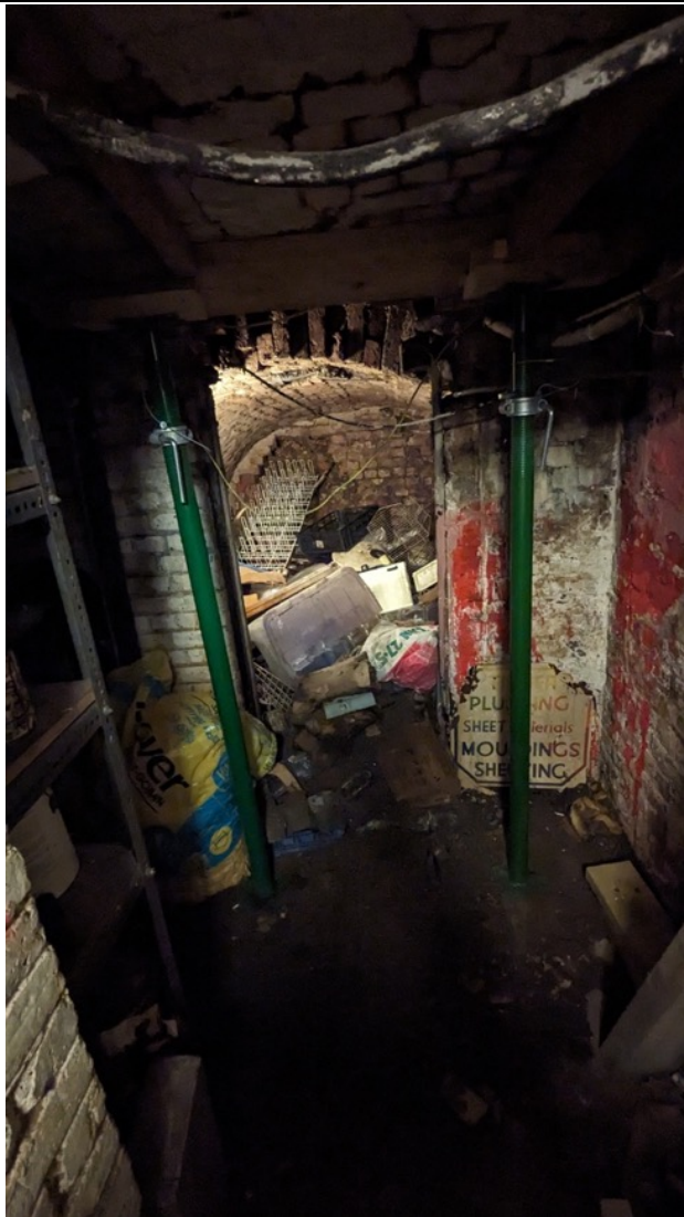
Photo 17: Brick wall at back of vault has collapsed exposing earth behind. Across temporarily installed to support collapsed ceiling of brick arch vault
