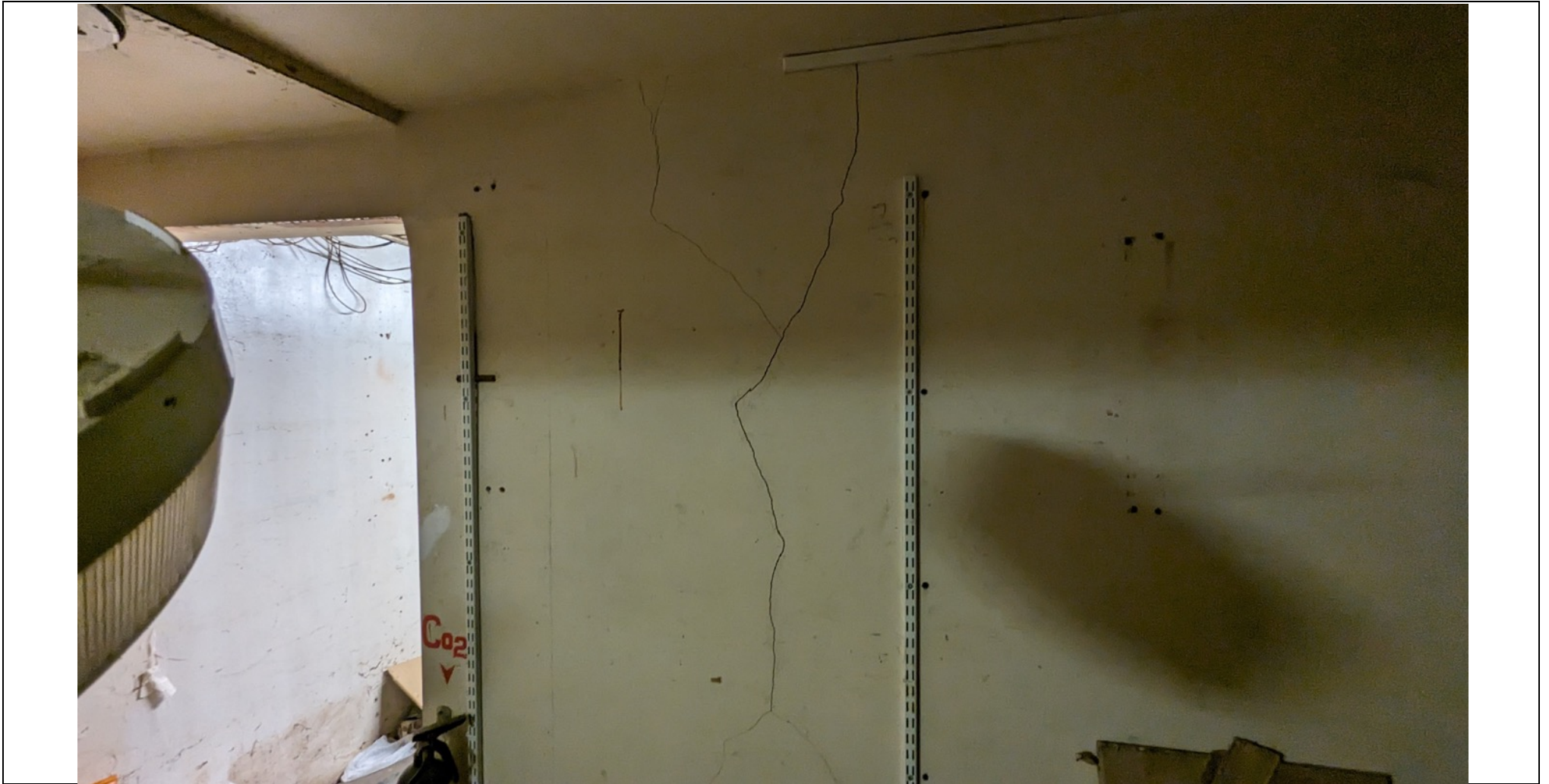
Photo 13: Cracking to central basement masonry wall
