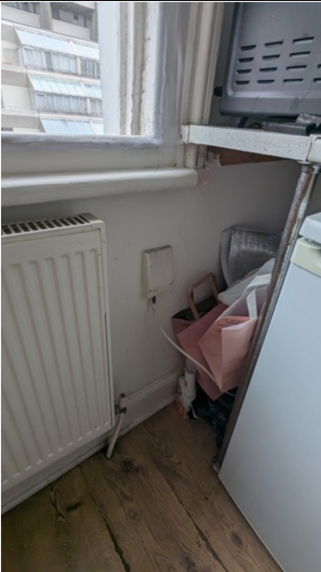
Photo 03: Second Floor flat (front elevation) showing crack from corner of window to floor
