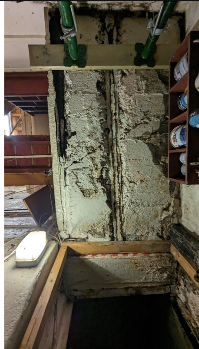
Photo 18: Across temporarily installed to support failed filler joist floor above basement
