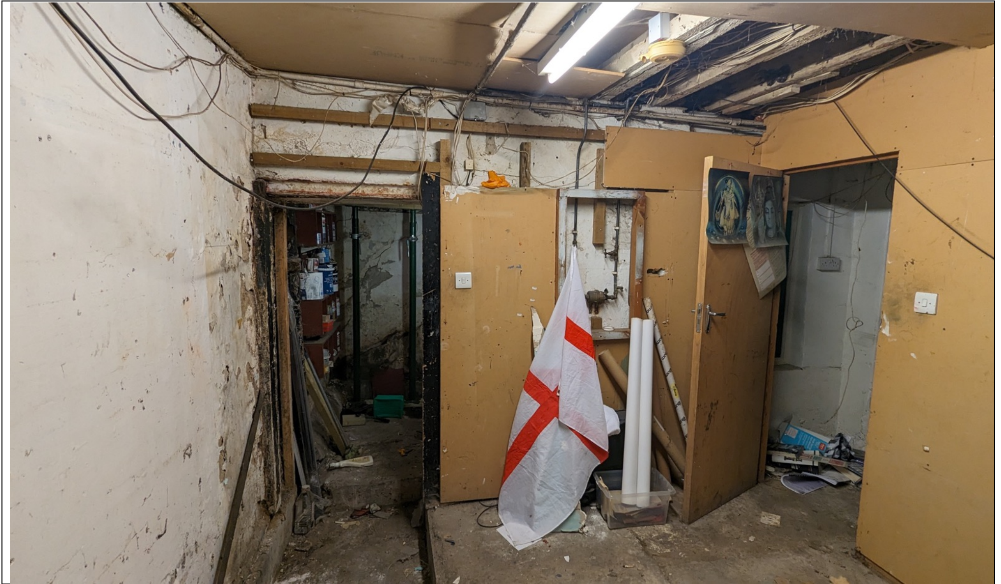
Photo 14: Rear wall of basement space. Cracking observed behind wooden panels horizontally and continues over top of door
