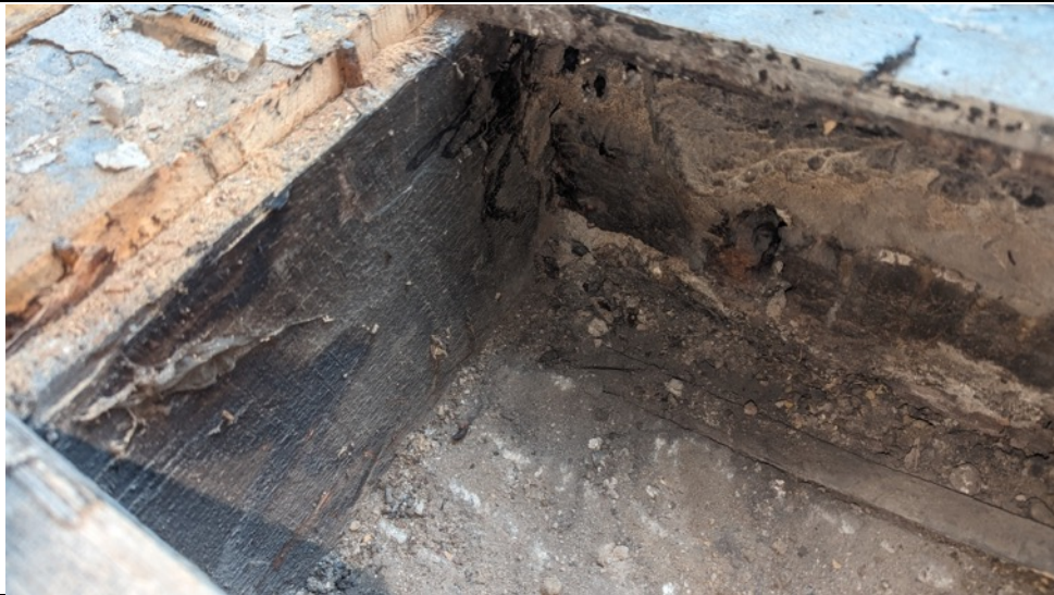
Photo 29: View of first floor timber joists after lifting floorboards at rear of property.
