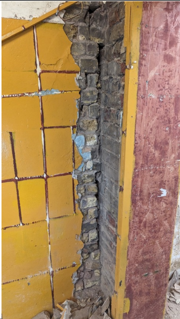
Photo 27: Spine wall at ground floor rear of shop is de-bonded from the party wall. Repair required
