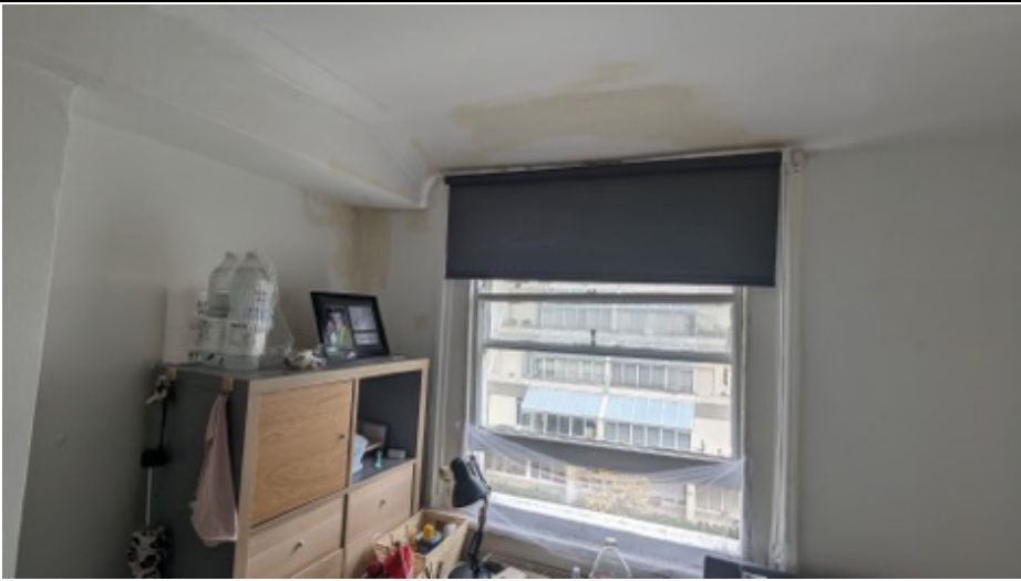
Photo 05: Top floor flat (front elevation) showing water damage to ceiling
