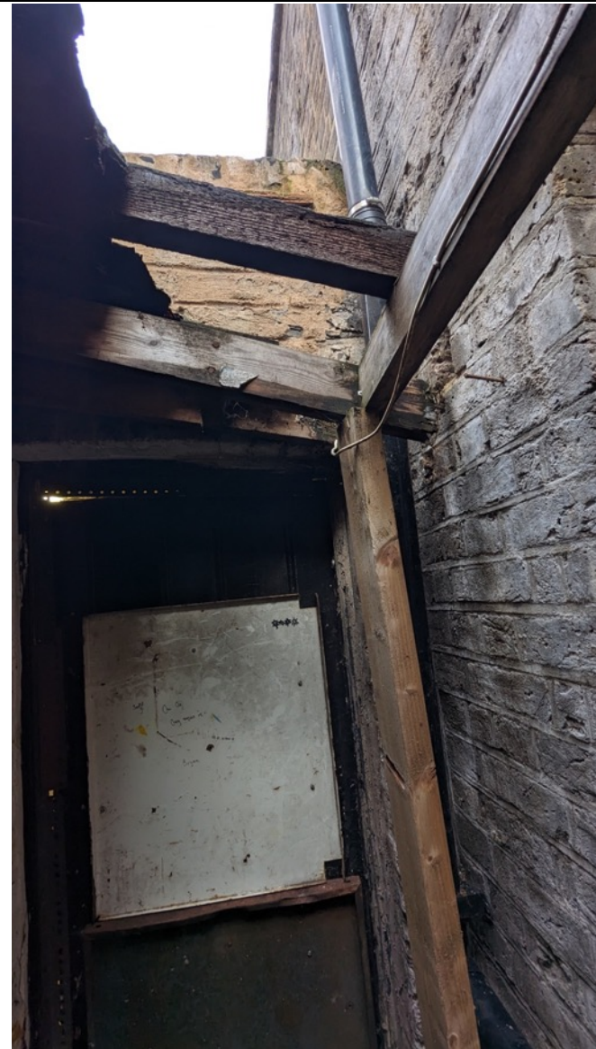
Photo 12: Delapidated timber roof structure over courtyard. Roof coverings missing in places
