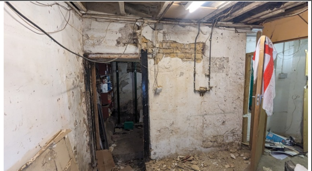
Photo 26: Rear wall of basement space. Removal of plaster shows various different brick types and historic interventions. Repair required
