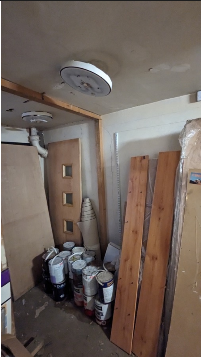
Photo 15: Vertical crack in wall to front of basement, extends to the horizontal position just below ceiling level
