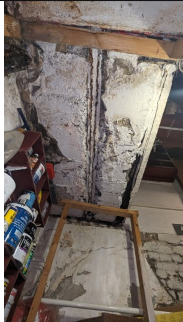
Photo 10: Corroding steels / filler joist floor, partially supported on temporary timber
