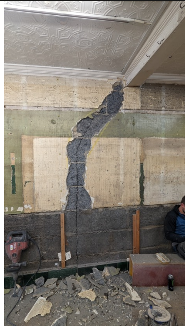
Photo 28: Ground floor wall separating the corridor and the shop unit, crack manifests through the plaster into the blockwork. Repair required
