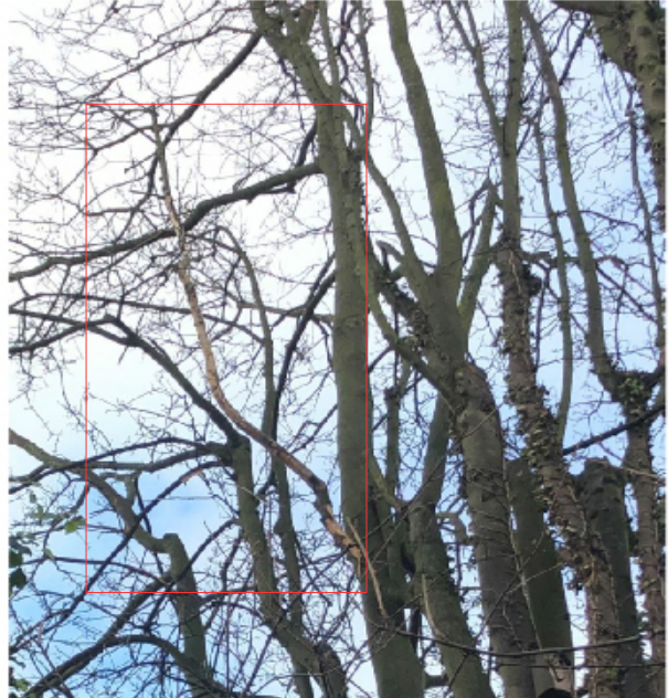
Major sized deadwood in the crown of T2 and overhanging the neighbouring garden to the west.
