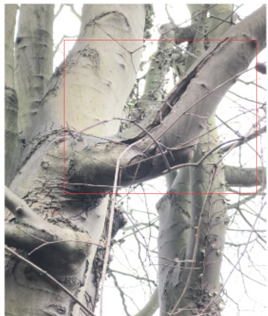
Close up photo of the Hazard Beam split limb on the north side of T2 at approx. 4m
