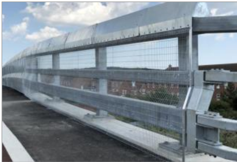
Figure 17 A case study image illustrating how the temporary parapet is expected to look (model shown is Varley and Gulliver VGSH 4000 H4a Parapet)
