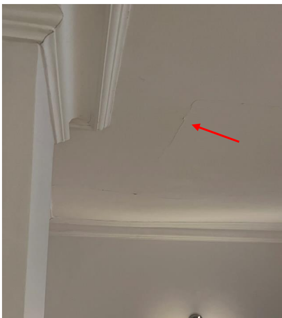
Photograph 13 – Cracking to ceiling
