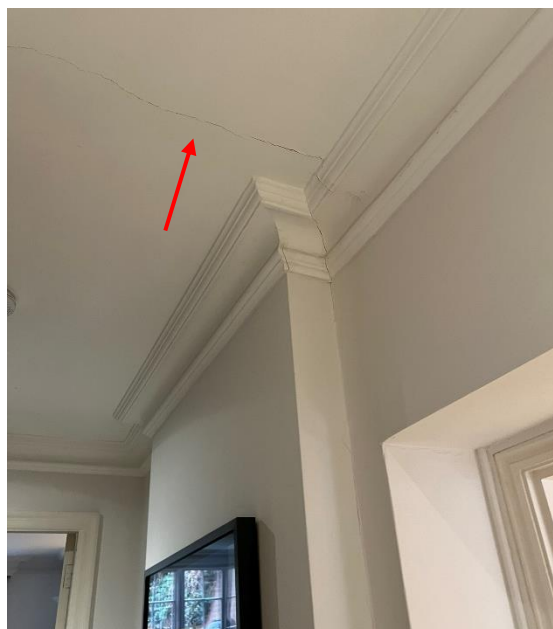
Photograph 14 – Cracking to ceiling
