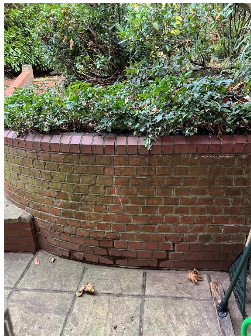
Photograph 6 – Cracking to retaining wall
