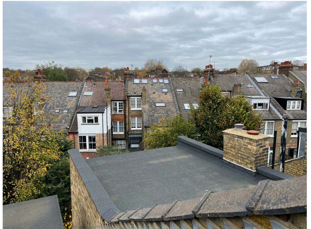
view showing flat roof to rear of No 16, with various rooflights on other neighbouring buildings (note this is looking at the rear of the Eastern side of Glenloch Road)
