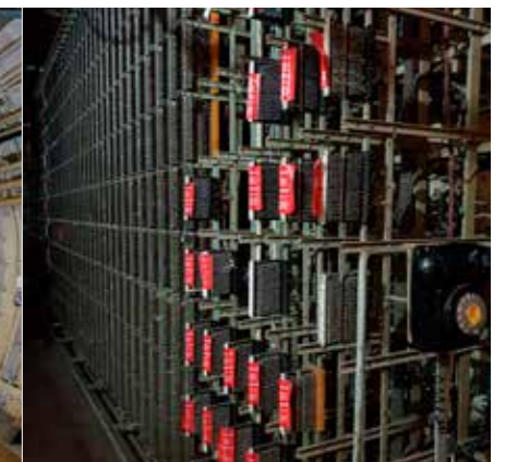
4 Main Distribution Frame
