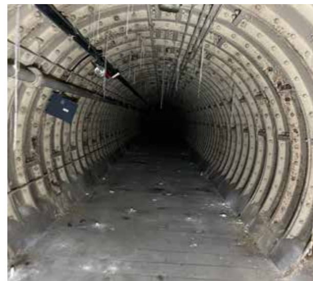
Cast iron lining
