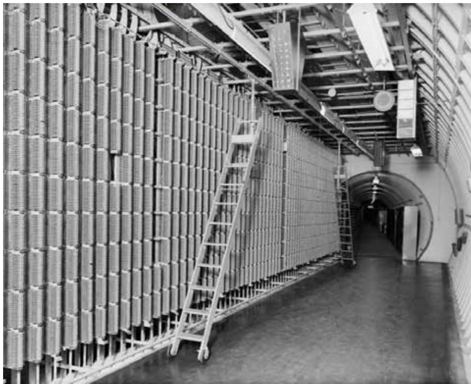
Figure 25. Telephone Exchange Main Frame -1950s
