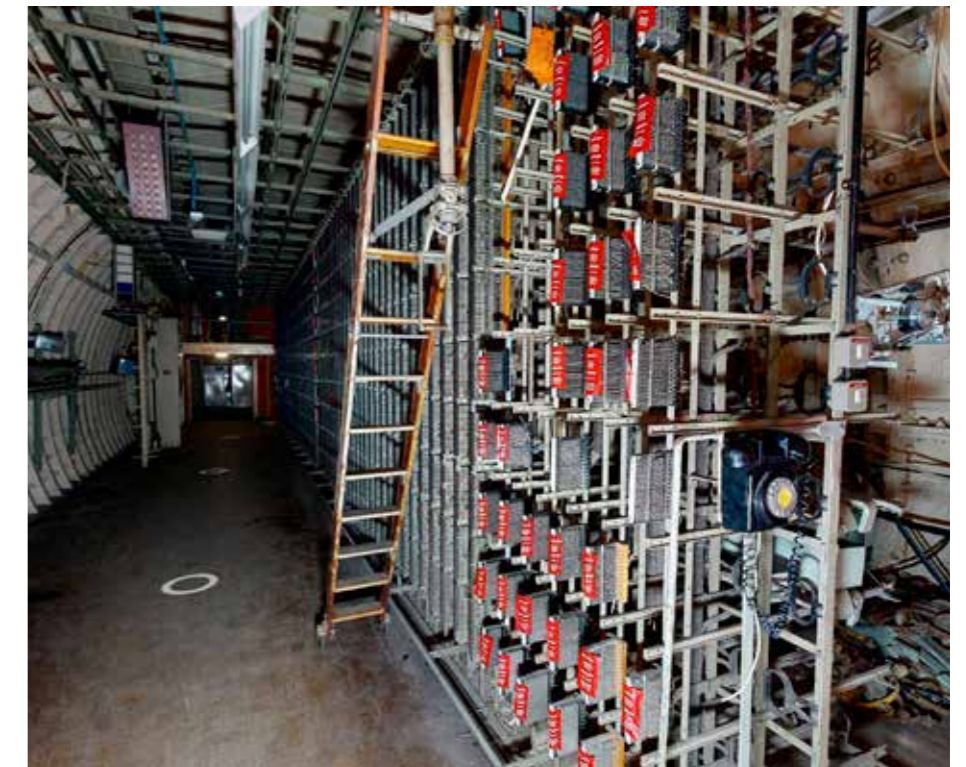
6 Telephone Main Distribution Frame
