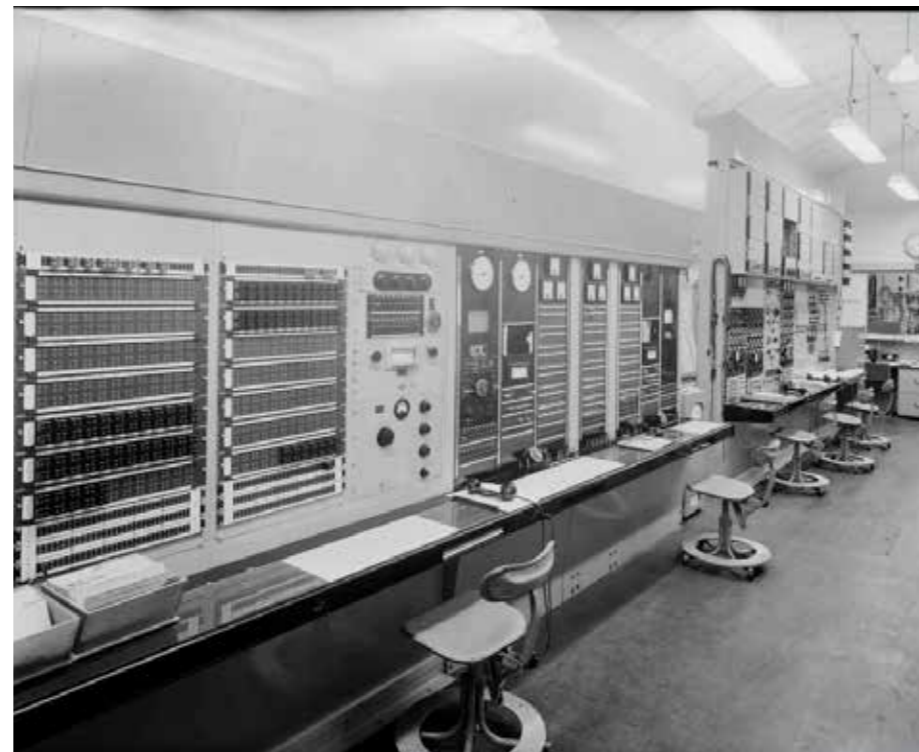
Figure 26. BT Archive - Operations room - 1950s
