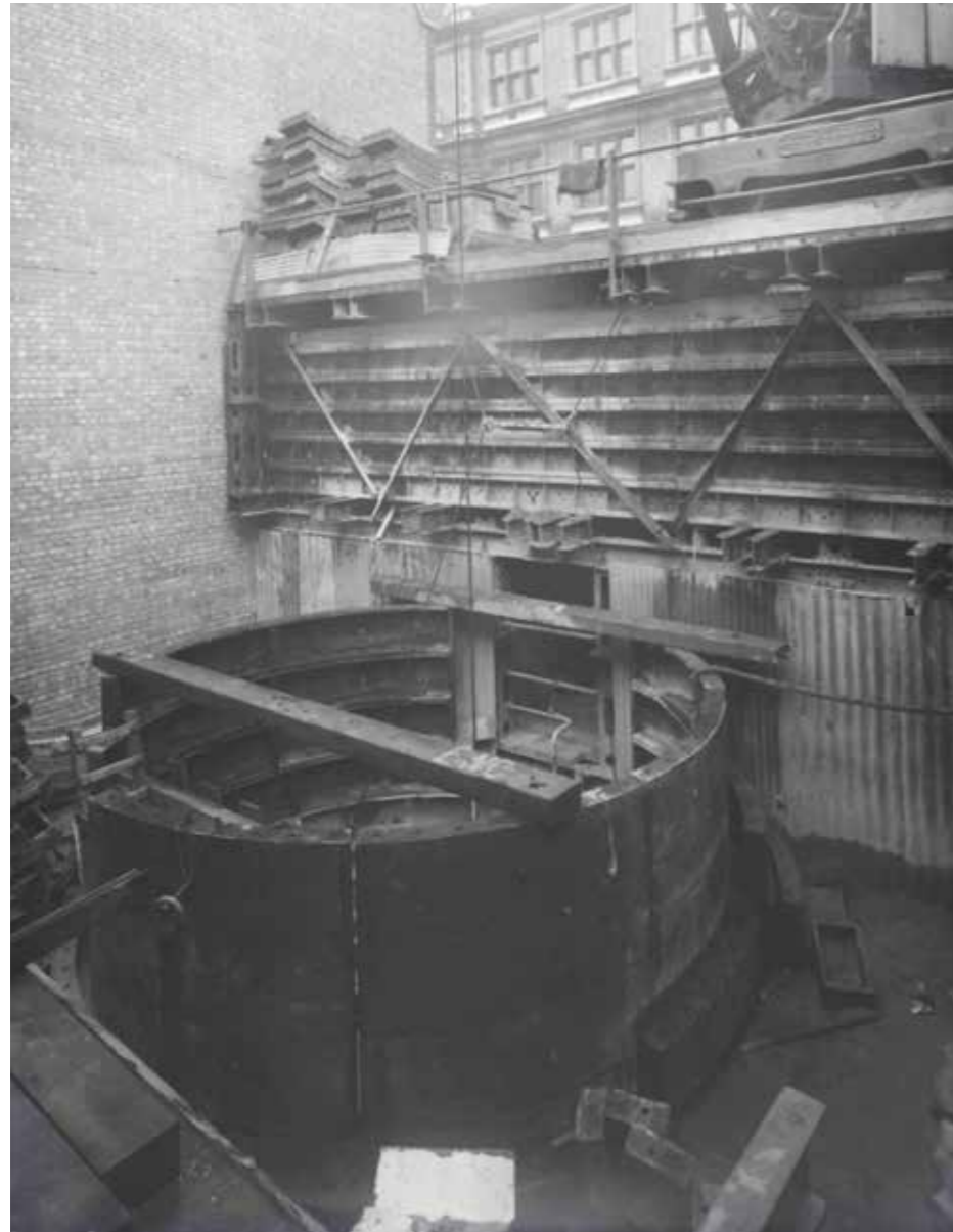
Figure 4.6 Construction of the goods shaft and No. 39 Furnival Street, 1952 (source: BT Archive)
