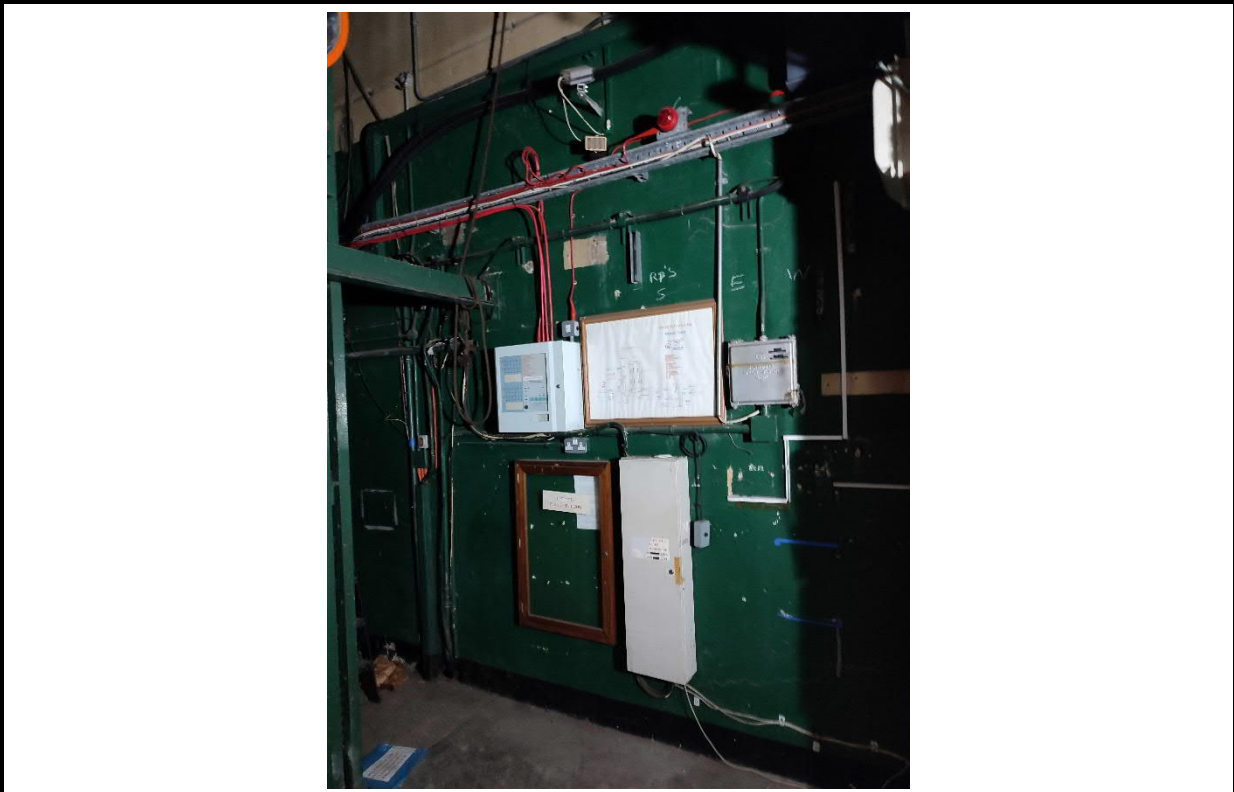
Photo 13: Photo of the southern interior wall of 38-39 Furnival Street from just inside the access doorway.
