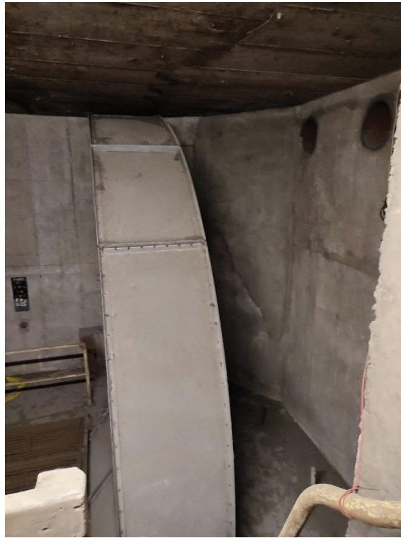
Photo 9: View down onto the shaft roof and ventilation grate on the centre and south side of the room, photo taken looking east.
