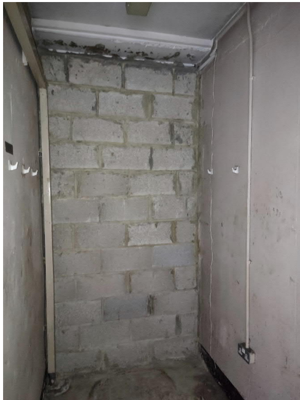
Photo 16: Photo of the bricked-up entrance located behind the black doors on frontage of 38-39 Furnival Street (see Photo 11).
