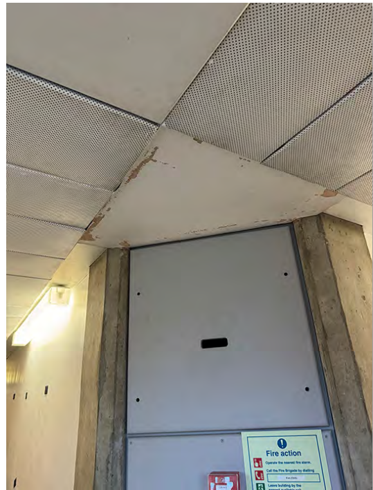
IMG_0760 Access panels to service riser
