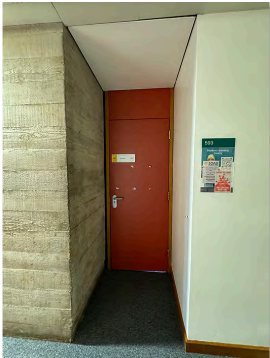
IMG_0780 Later addition plastic laminate faced door and over panel to Room P593
