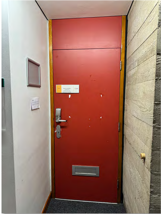
IMG_0776 Later addition plastic laminate faced door and over panel to Room P579
