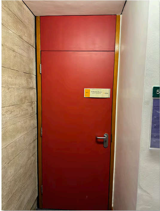
IMG_0766 Later addition plastic laminate faced door and over panel to Room P571
