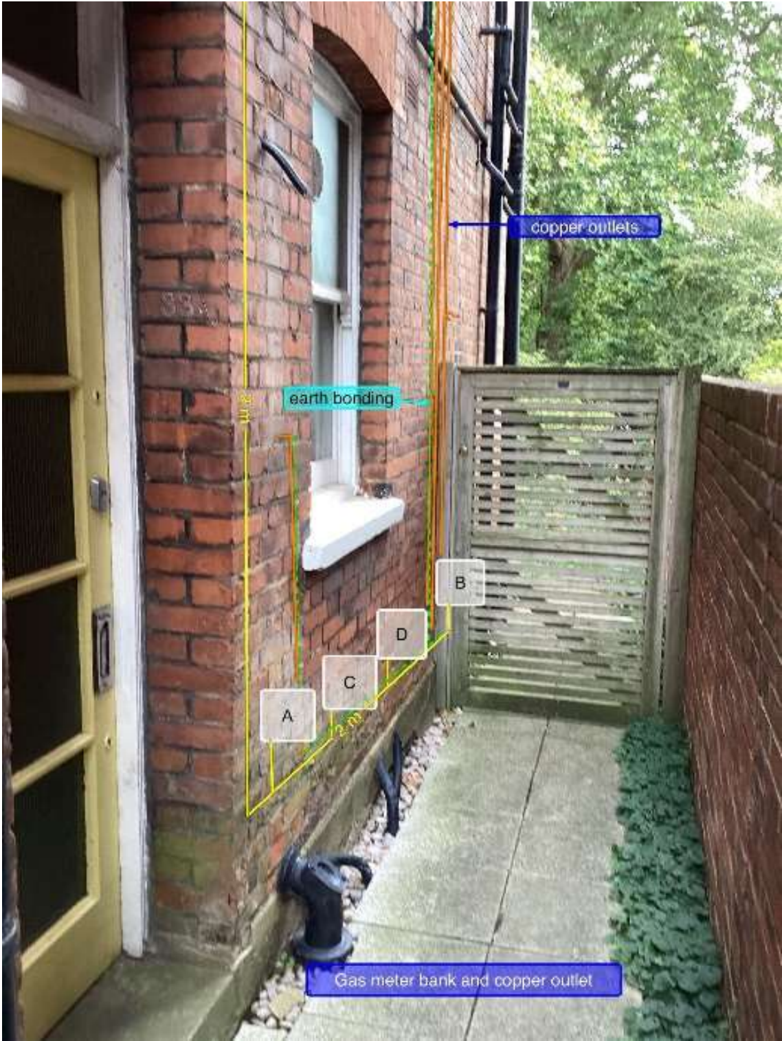
Figure 4 Proposed location of the 4 no. new meter boxes to the side elevation.
