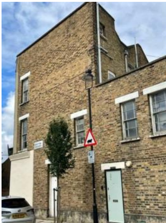
Figure 13: Photo taken at south end of Grafton Crescent, showing broken valley roof, visible at street level.
