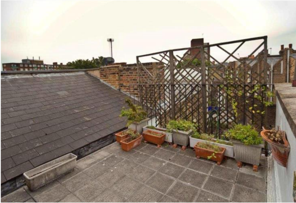
Figure 16: Roof terrace and broken valley adjacent No. 14.
