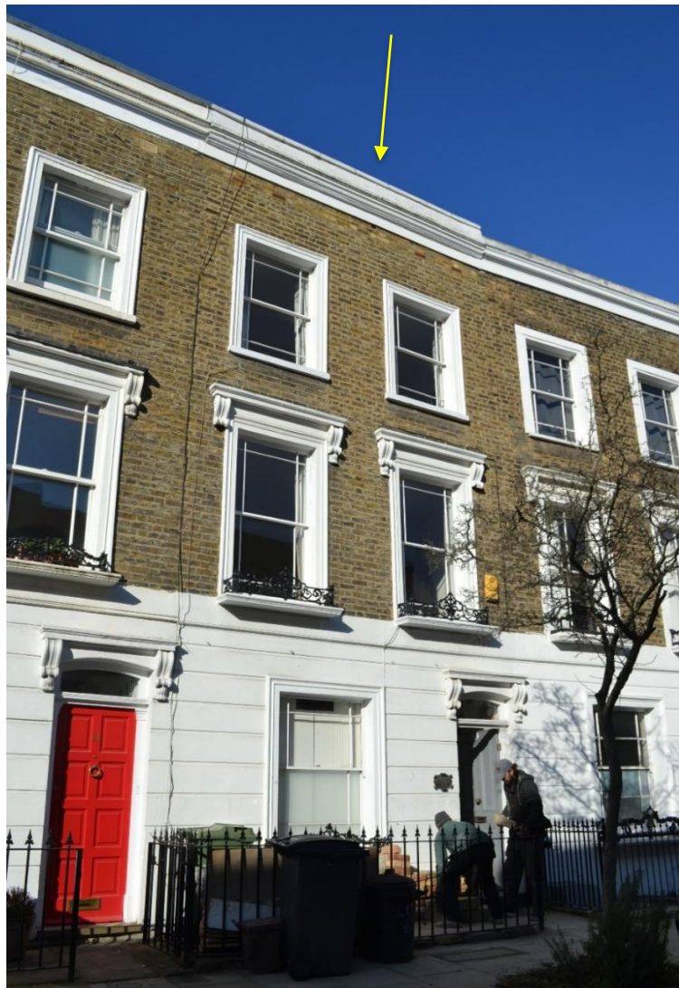
Figure 8: Front elevation of No.13 Grafton Crescent- note the varying profile of the parapet (highlighted in yellow).
