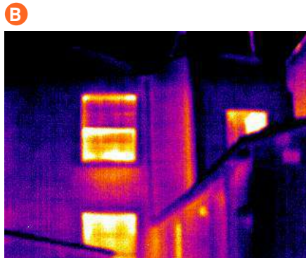
B Heat from internal radiators beneath the windows. The proposed retrofit includes for all existing walls be internally insulated.
