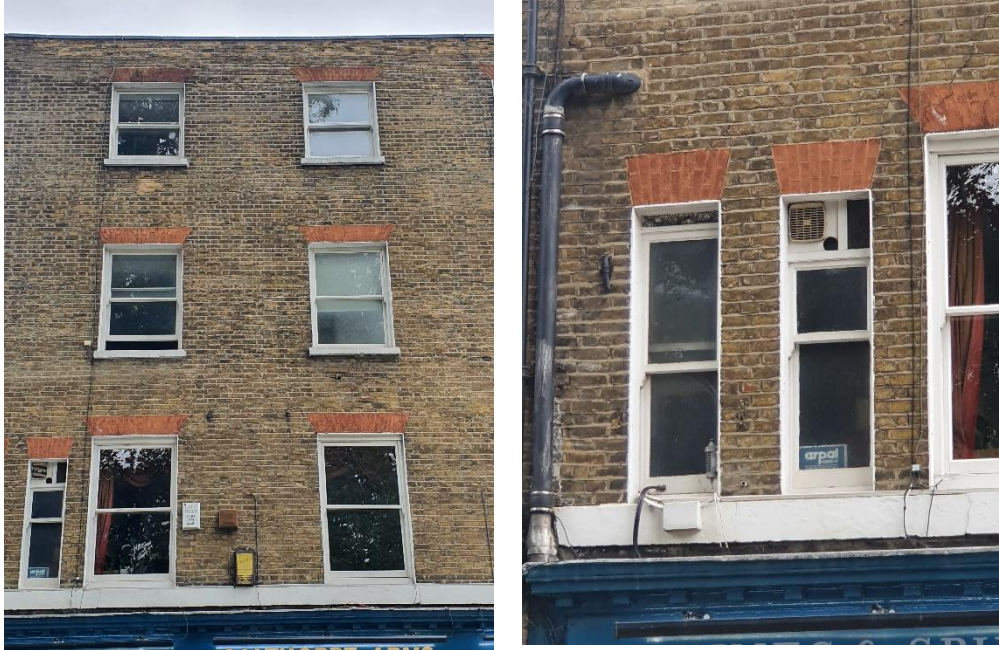
Fig 11 and 12: View of site from Wren Street, facing South East – focusing on existing window composition
