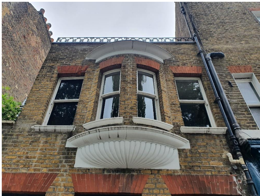
Fig 7: View of site from Wren Street, looking up at existing oriel window
