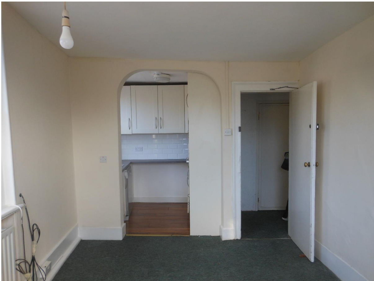
Fig. 15: Third-floor living room and kitchen. The basket arched opening to the kitchen is modern and the partition to the right is a modern insertion (as seen by the way it cut across the architrave of the door).
