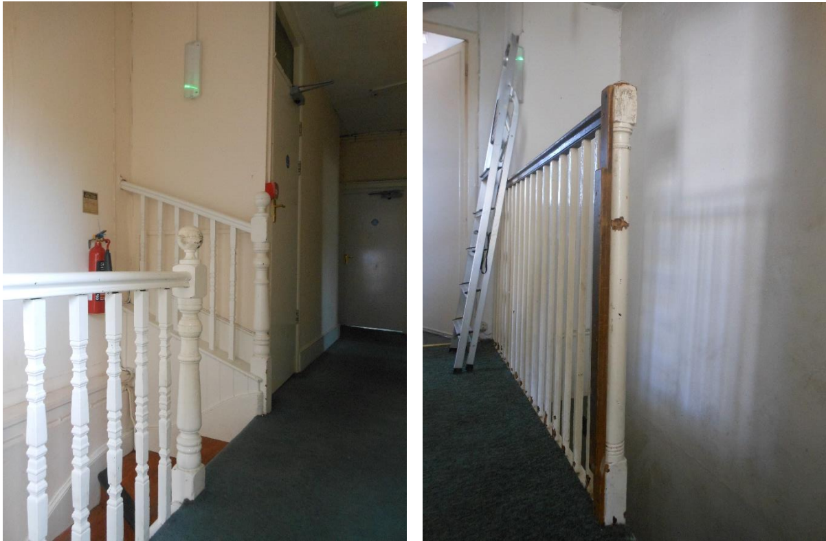
Fig. 14: Historic balustrades. Left to right: on the second floor (c.1900) and third floor (1820s) (18 January 2023).
