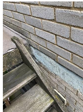
E.4 – External stair and exposed slab – significant thermal bridge.
