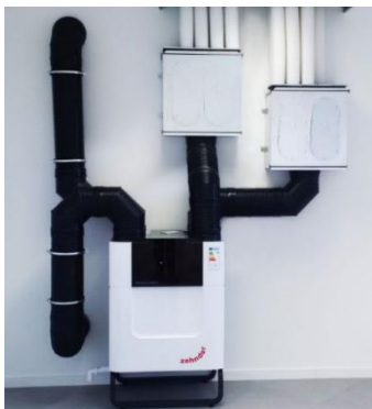
Zhender Comfowell MVHR Unit – Note duct manifold to to right and individual ducts to spaces.
