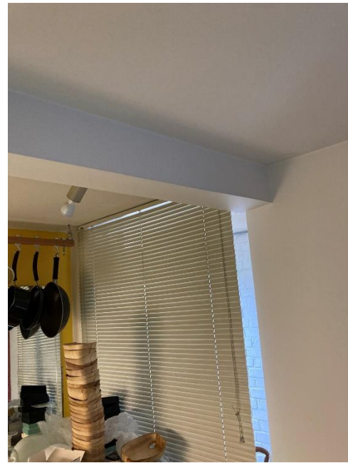
E.6 – Kitchen – beam is below slab height and windows extend to slab making distribution of services though voids difficult without reducing ceiling hieghts.
