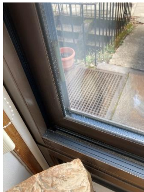
E.3 – Double glazing to front windows.
