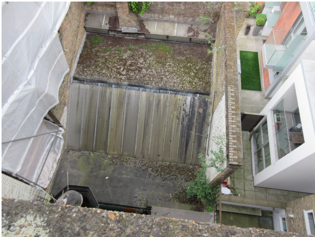
View of roof of existing rear extension (studio) with Crabtree Place to right
