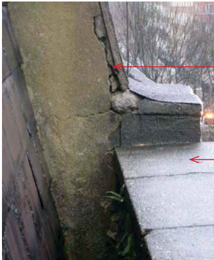
Broken & damaged render to party wall with no.42
