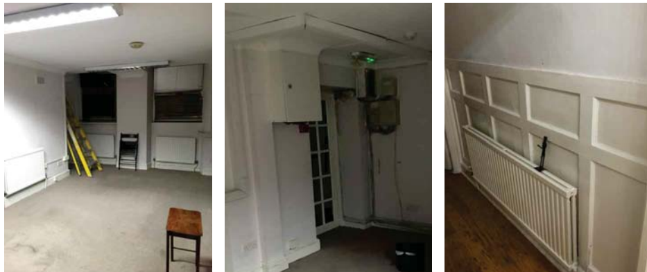
Examples of poorly integrated services throughout the house
