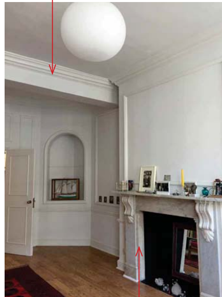
Non original fire surround
