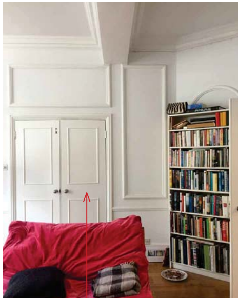
Non original door openings & panelling
