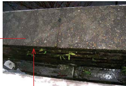
Concrete coping stone with no drip detail
