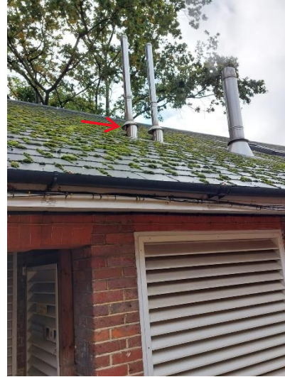
Plate 4.18: Flush Lead Flashing
