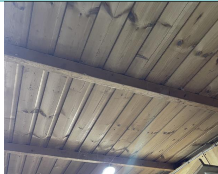
Image 34 Maintenance Shed - Timber Slates from Ceiling
