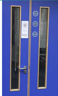
Image 54 GS Wing - Glass from Internal Doors
