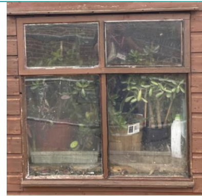
Image 51 Maintenance Shed - Single Glazed Window
