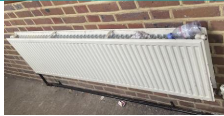
Image 15 Fives Courts - Steel Radiators
