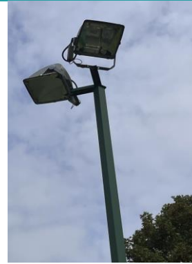
Image 24 External Areas - Steel from Lighting Column
