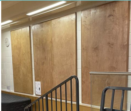
Image 41 GS Wing - Timber Wall Sound Insulation
