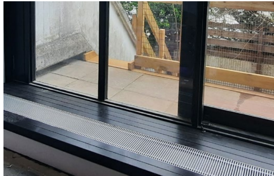
Plinth in living room of 46A pilot flat (B3 Flat Type) with integrated trench heater
