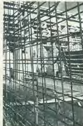
4 The heating coil can just be detected between the two skins of reinforcement.
