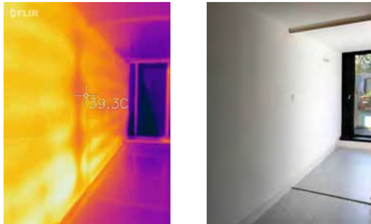
Figure 9: Internal image of a void A1 unit, showing the coil heated party wall - facing towards Rowley Way.
