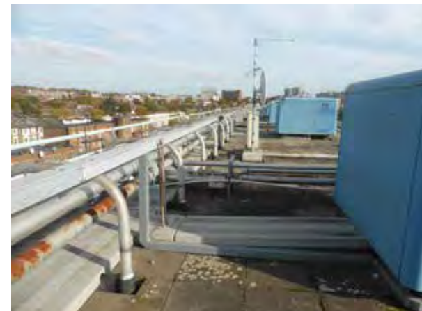
Figure 3.3 - Roof of block A showing distribution pipework and blue cold water tank pods
