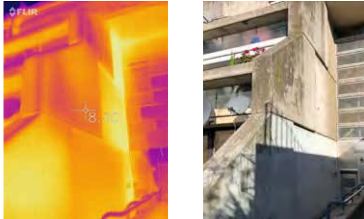
Figure 5 : Eastern end wall of block A illustrating heat loss from the flats. The thermal image was taken at 8pm to prevent the heat from the sun affecting the image. The photograph was taken the following day.
