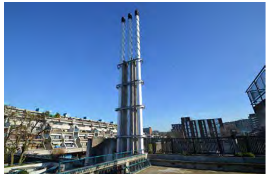
Figure 3.2 - Gas boiler flues rising from the boiler house
