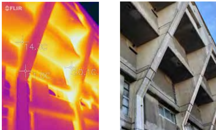
Figure 2: Rear of block A showing the heated party wall (right) and an unheated wall (left). The temperature readings from the image show that there are significant thermal bridges from the party walls. The unheated wall has a 3°C difference between the external wall (14°C) and the edge of the spine (11°C). The heated party wall (20°C) is 6°C warmer than the unheated wall (14°C).
