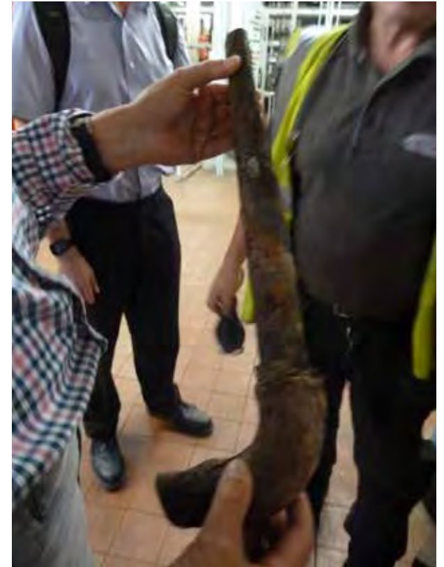
Figure 4.4 - Corroded pipework section
