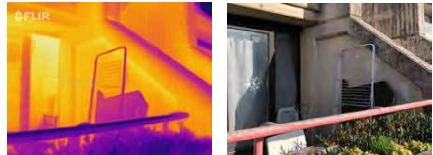
Figure 8 : Front of block A illustrating heat loss and the thermal bridge from the unheated party wall. This image shows that it was 3°C cooler on the unheated side (12°C) than the heated wall (15°C, figure 7) The thermal image was taken at 8pm to prevent the heat from the sun affecting the image. The photograph was taken the following day.
