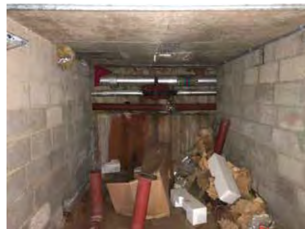
Figure 3.4 - Garage under block B showing distribution pipework along the back wall
