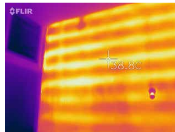
Figure 3.7 - Thermal image of a heated wall coil in block A, showing a surface temperature of 38°C
