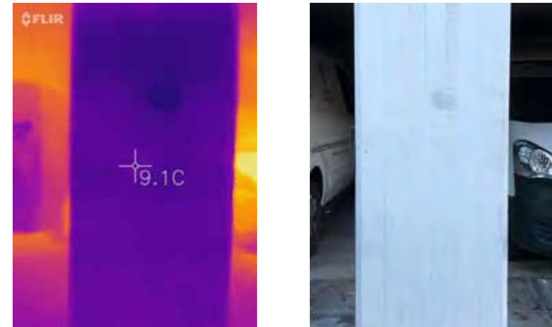
Figure 3: The base of the spine wall between the parking spaces at the ground floor of block A was measured at 9°C. This shows that the thermal bridge from the flats extends to the edge of the spines with a 2°C difference between the lower (9°C) areas and upper floors (11°C).
