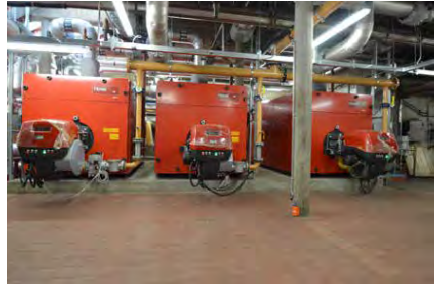
Figure 3.1 - Gas boilers in the boiler house
