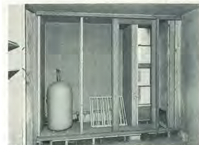
5 Cupboard unit against the wall beside the railway provides additional sound resistance. The calorifier acts as a heat exchanger for domestic hot water. Under the cupboard is the fresh air inlet convector with a long shunt duct to reduce noise from outside. The window reveal covered by a sliding glass door acts as a deep double glazed unit. Note the tapering scribed timber at high level due to tolerance difficulties.
