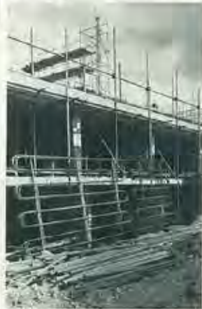
3 The prefabricated heating coils are stacked ready for placing in the cross walls.
