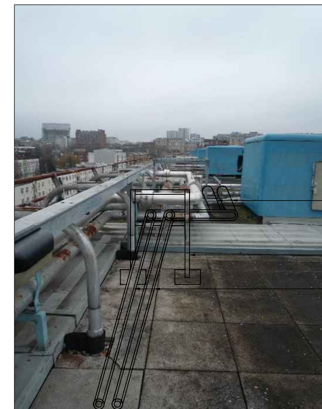
PROPOSED PARALLEL HEATING INSTALL (ROOF LEVEL) PHOTO REF P1
