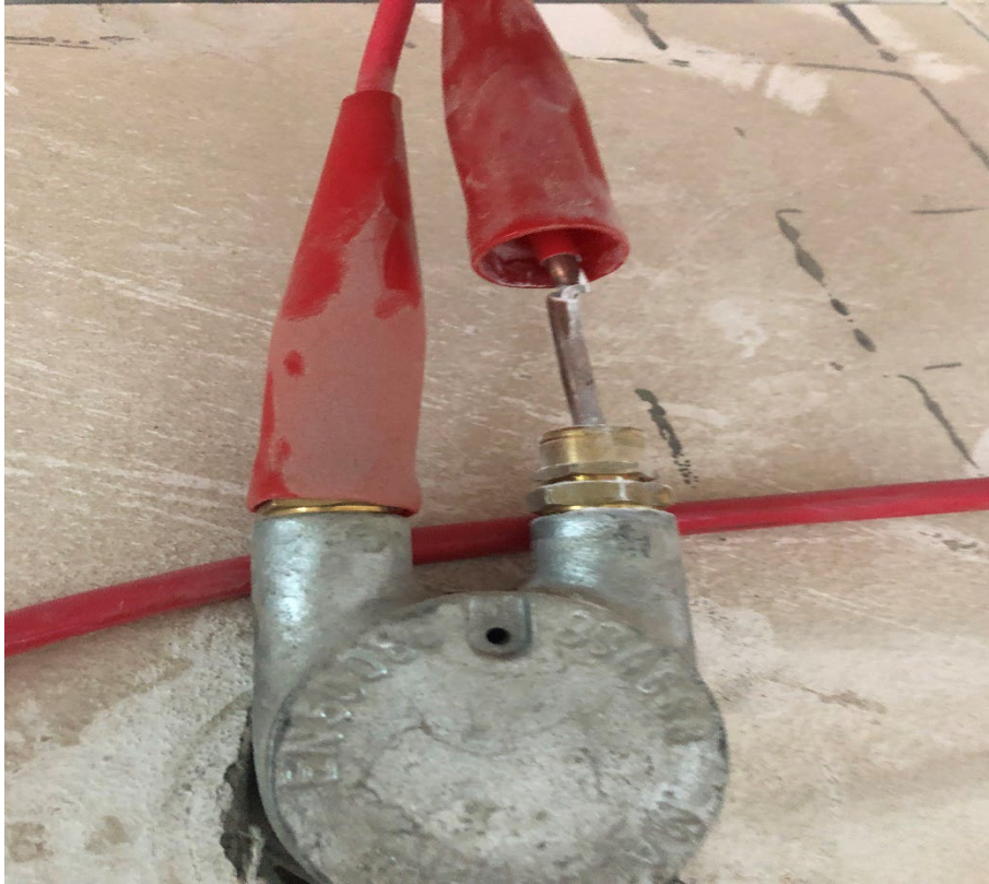
Damaged pyro causing short circuit on level 32
