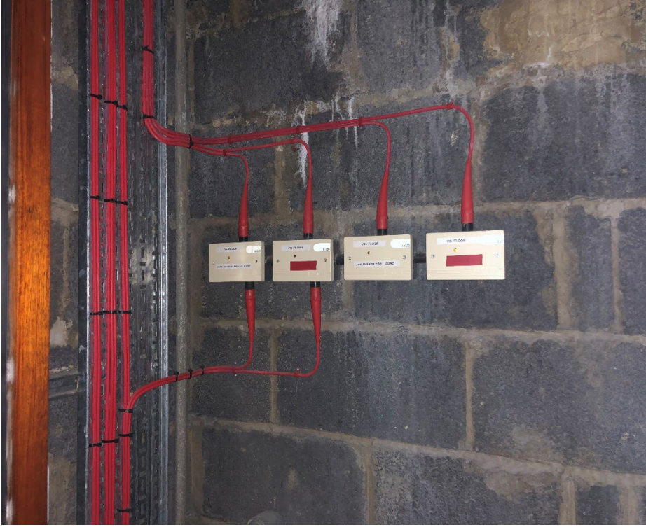
Isolators from old risers installed on most floors as using as feed wiring for the loops on each floor.
