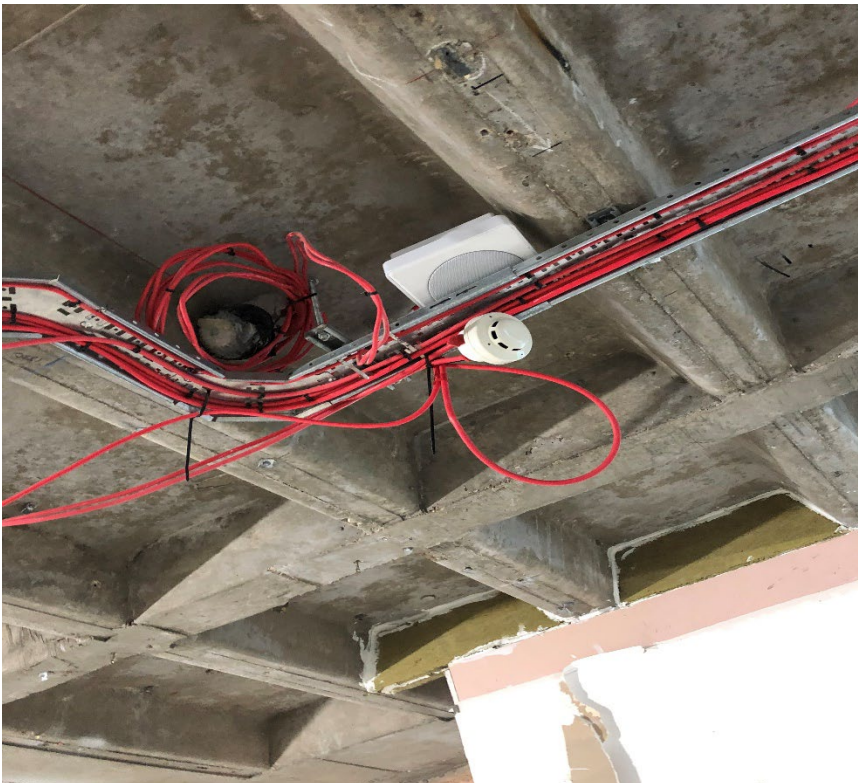
Old Cabling / Smoke from previous system.
