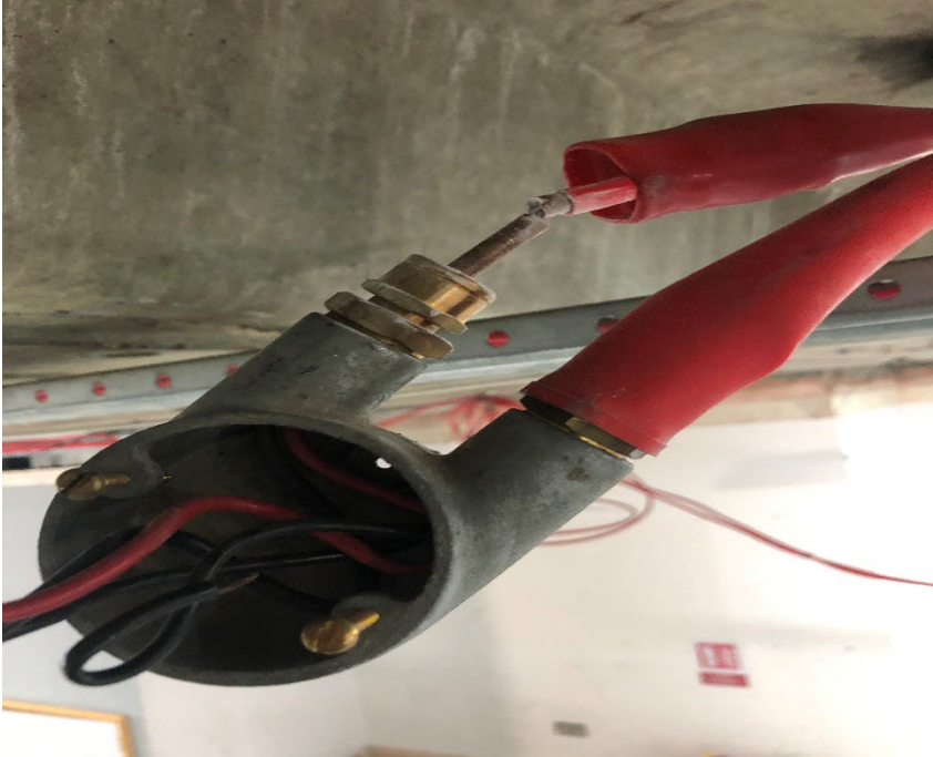
Pyro cable damaged causing short circuit on loop, Level 28
