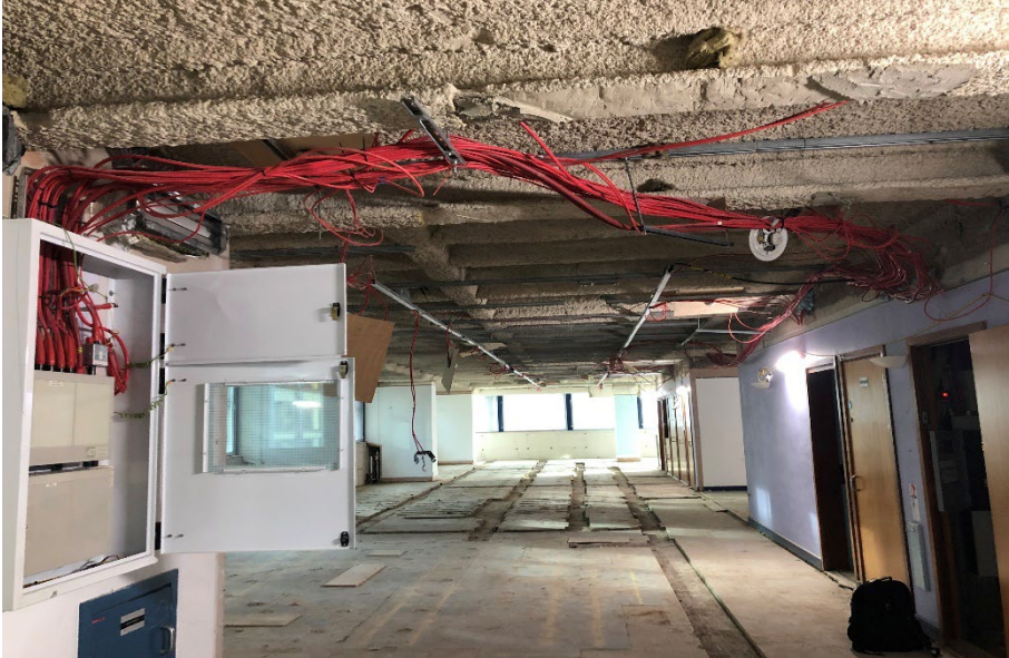
Level 3 – Old FA system panel used as JB to feed loops for new gent system / panel in adj riser.
