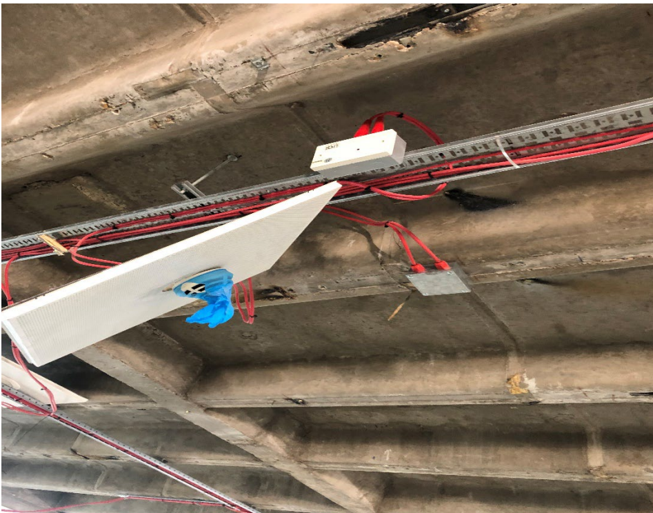
Multiple joint boxes and old zone isolators across all floors.
