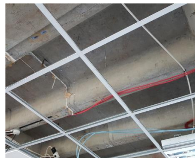
Figure 2: Soffit of Level 17 slab as-struck concrete ribs with some cast-in channels and some surface-fixed services (image courtesy of 190925 ARUP Invasive Survey Report)
