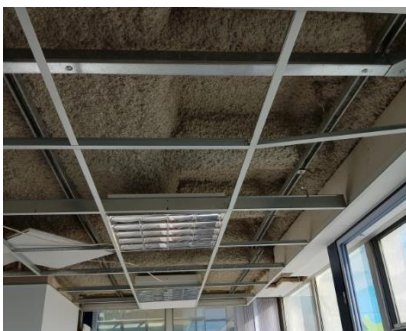
Figure 1: Soffit of Level 5 slab showing sprayed material on ribbed slab applied around ceiling and services supports (image courtesy of 190925 ARUP Invasive Survey Report)
