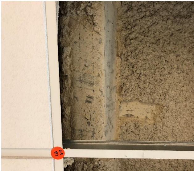
Figure 10: Level 4 East spur – large area of SFRM removed for CVI by others as part of the structural investigation
