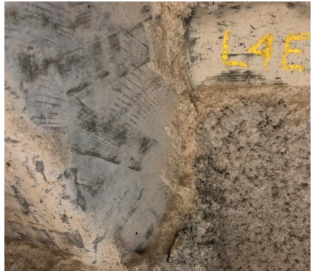
Figure 11: Level 4 East spur showing the cohesive failure of the SFRM on removal with mechanical tools – indicating good adhesion
