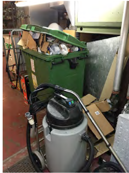
Combustibles in plant room.
