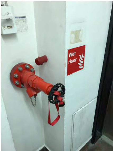
Straps need installed correctly
