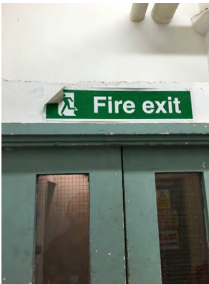
Some signage is peeling away and should be repaired or replaced.
