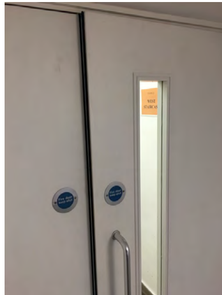
Some doors not closing fully due to faulty self closers
