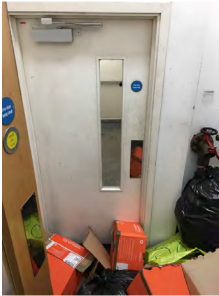
Rubbish blocking means of escape
