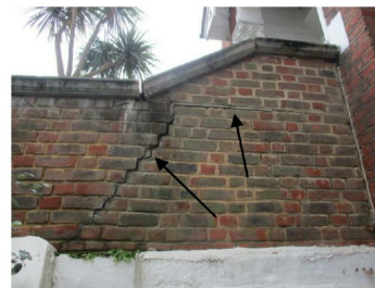
Cracking to right hand side steps wall
