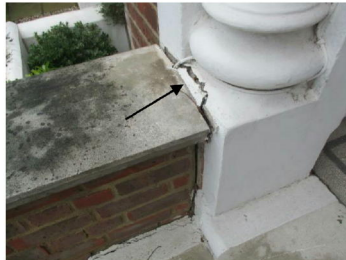
View of cracking to front steps
