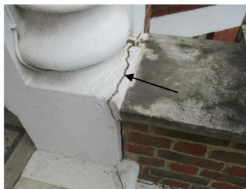
View of cracking to front steps
