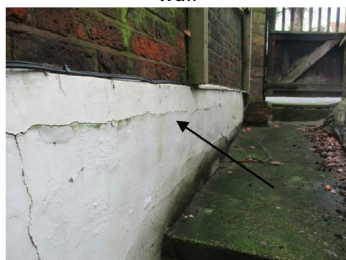
View of bulging and cracking to right hand boundary wall
