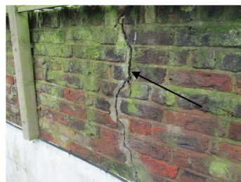
Cracking to right hand boundary wall
