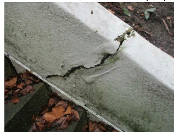
Cracking to retaining wall
