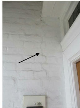
View of cracking to porch
