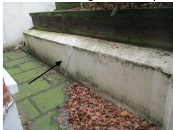
View of cracking and leaning to retaining wall
