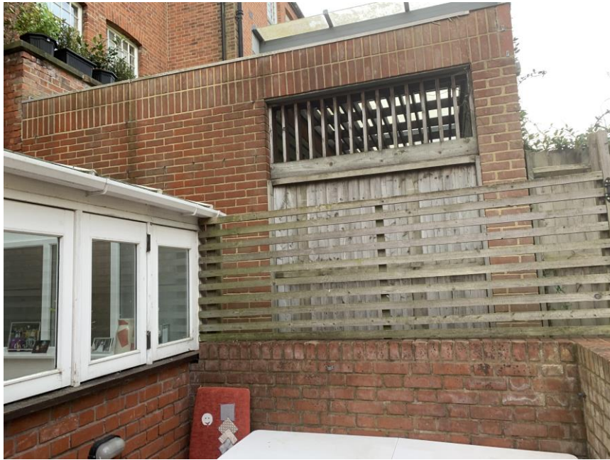
P2: Extension of No 14 Wedderburn Road and relationship with existing building line of application site.
