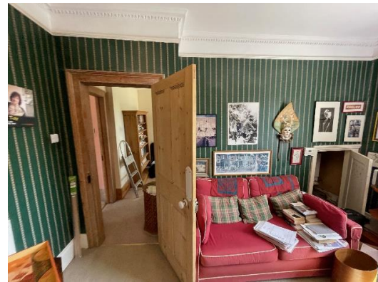
Figure 18: A view within the rear room looking towards the inserted partition and lobby.
