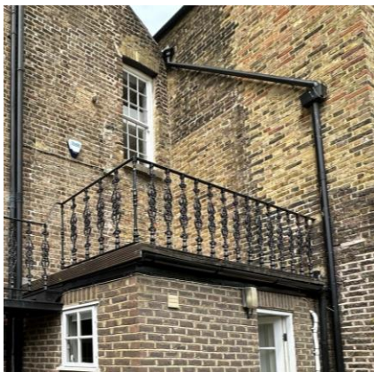
Figure 5: The scar on the brickwork flan of no.43 Downshire Hill.
