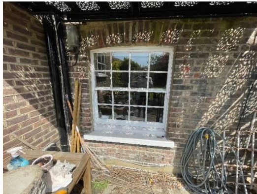
Figure 22: The existing replacement sash window to the rear room at basement level.
