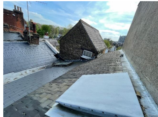
Figure 24: The existing roof slope to the entrance bay looking out of the existing 2 nd floor side window.
