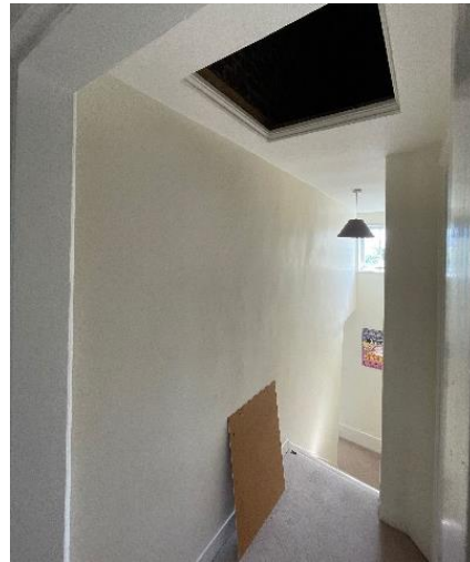
Figure 26: The wall where the new window opening will be installed at 2 nd floor level.
