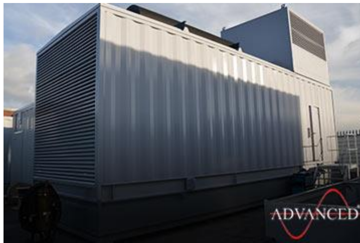
Figure 16 Typical container type generator (roof mounted intake)
