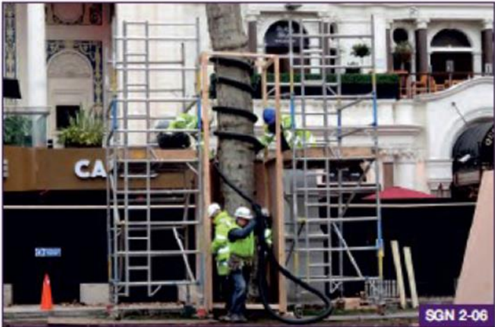
Improvised use of drainage pipe wrapped around the trunk can provide an added layer of protection beneath a layer of plywood.
