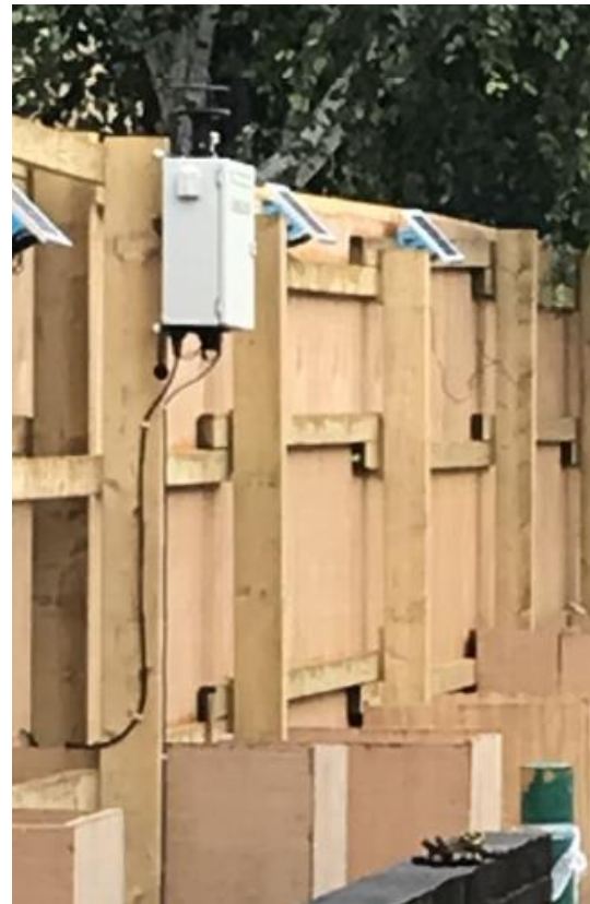
Noise, Dust and Movement Monitoring Station
