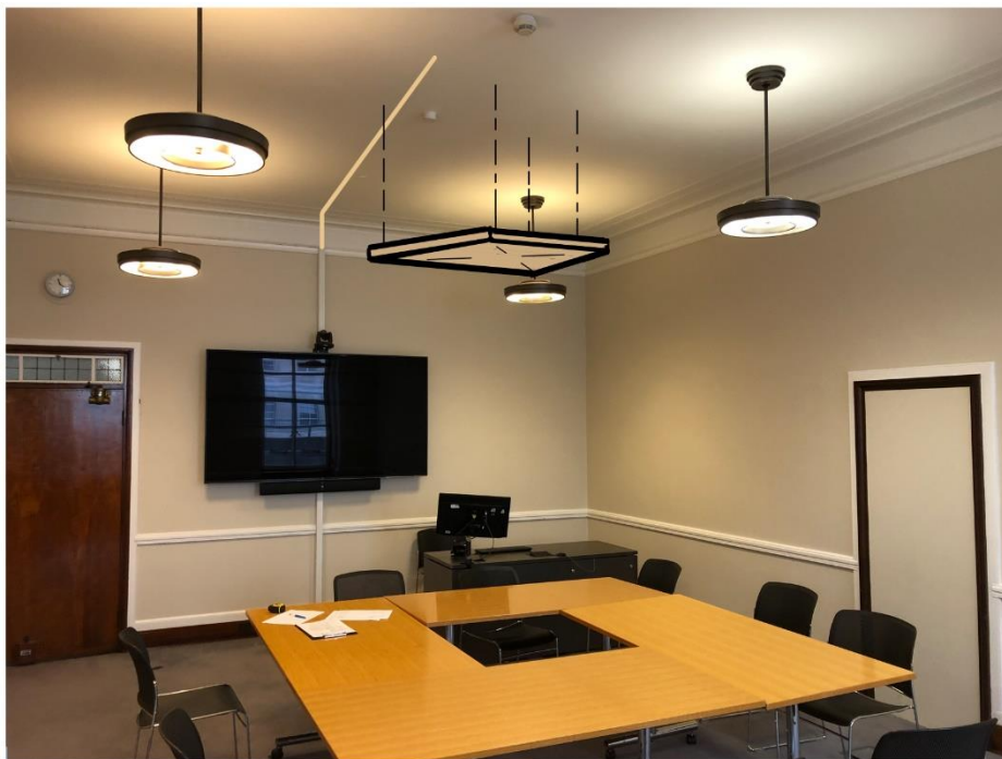
New microphone suspended from ceiling and proposed new containment.
