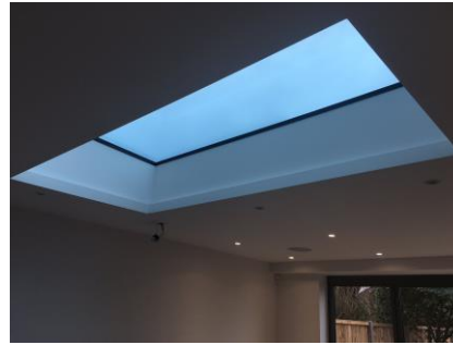
Photo showing example of skylight with obscured glazing
