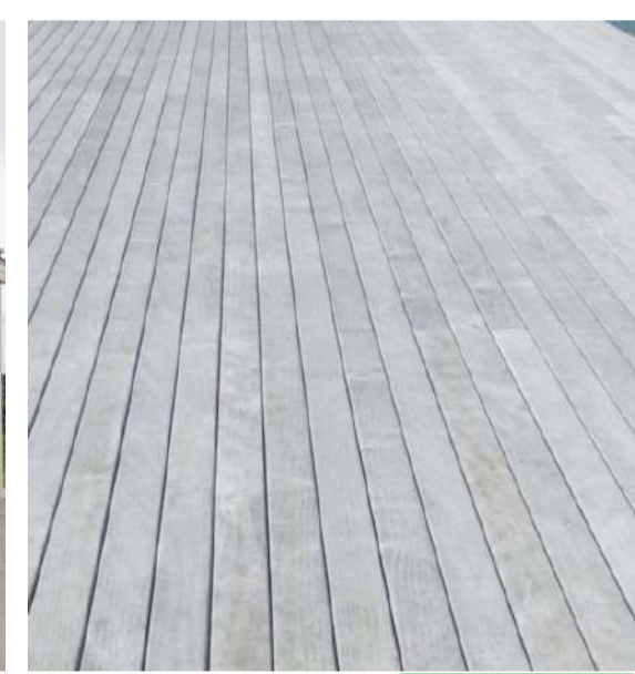
ACCOYA CLADDING AFFECTED BY SUNLIGHT
