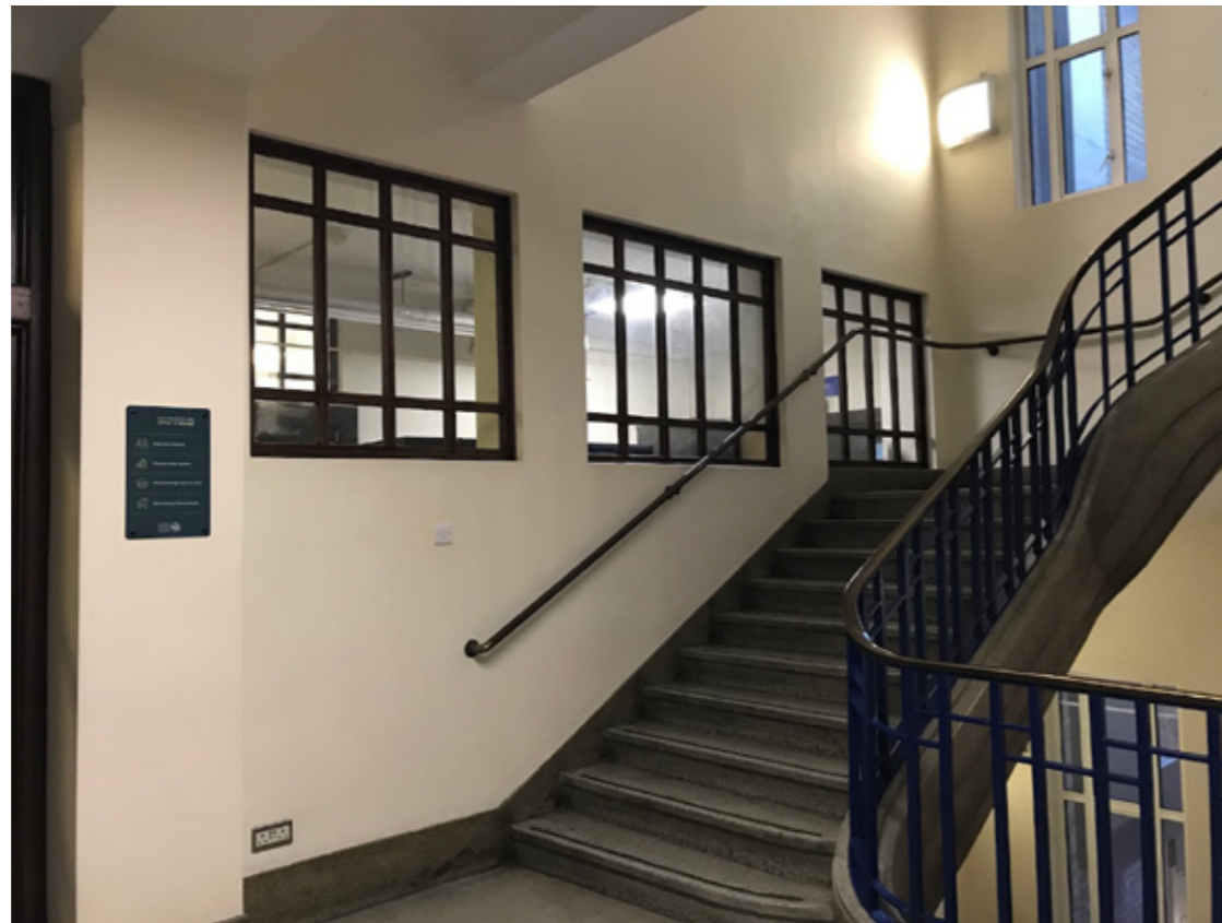
Photograph P6: Stair Core 2 North-East Elevation: Existing Windows at Third Floor (Stair Core Side)
