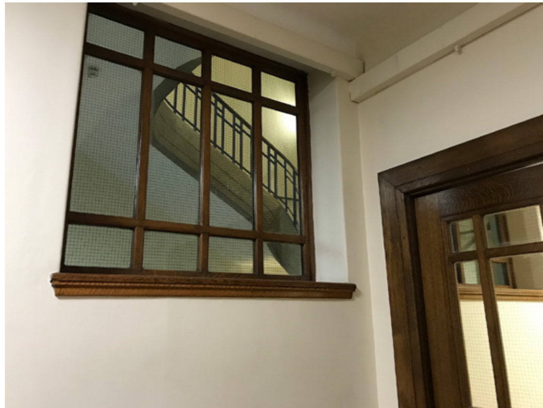
Photograph P6: Stair Core 3 South-West Elevation: Existing Windows at First Floor (Corridor Side)
