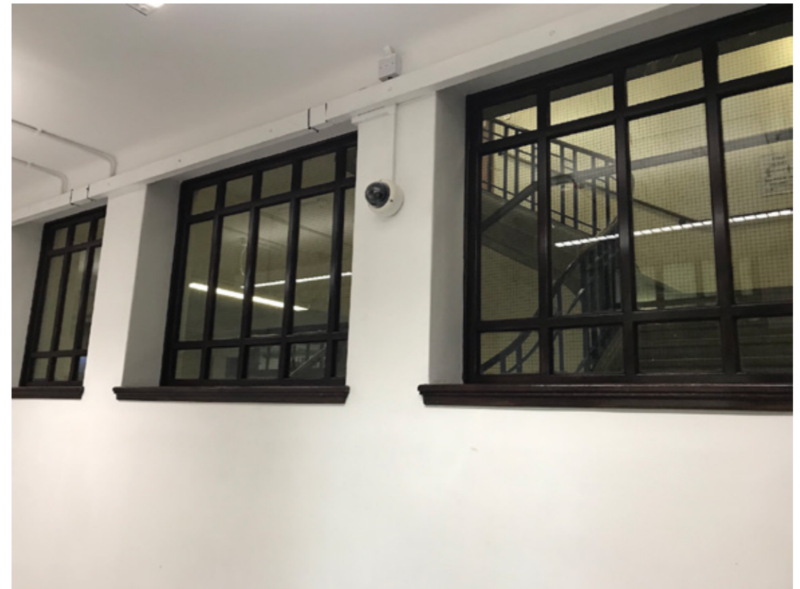
Photograph P6: Stair Core 3 South-West Elevation: Existing Windows at Third Floor (Corridor Side)
