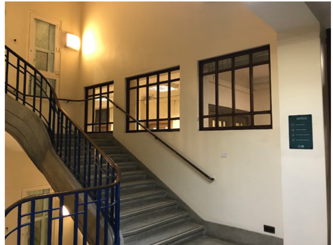
Photograph P5: Stair Core 3 South-West Elevation: Existing Windows at First Floor (Stair Core Side)
