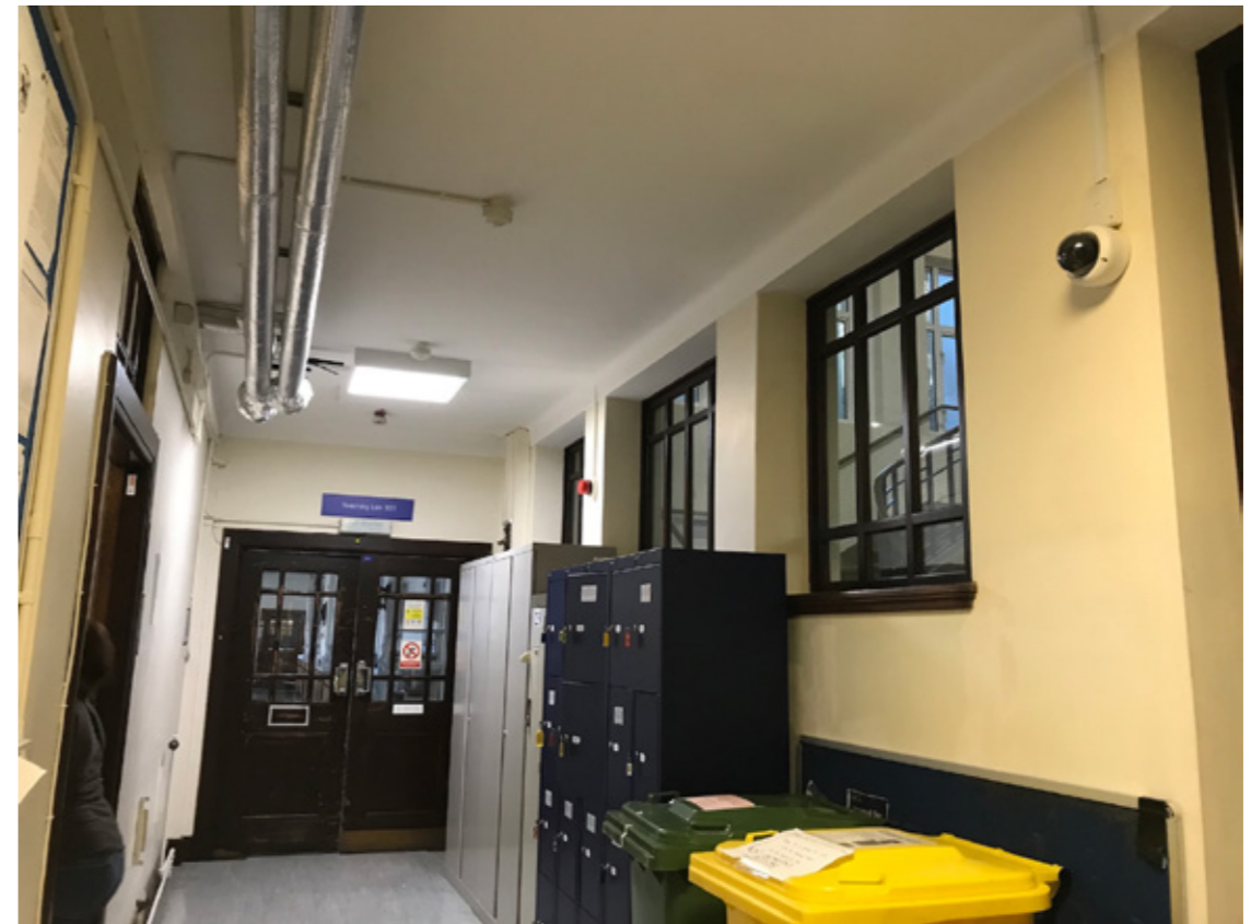
Photograph P7: Stair Core 2 North-East Elevation: Existing Windows at Third Floor (Corridor Side)
