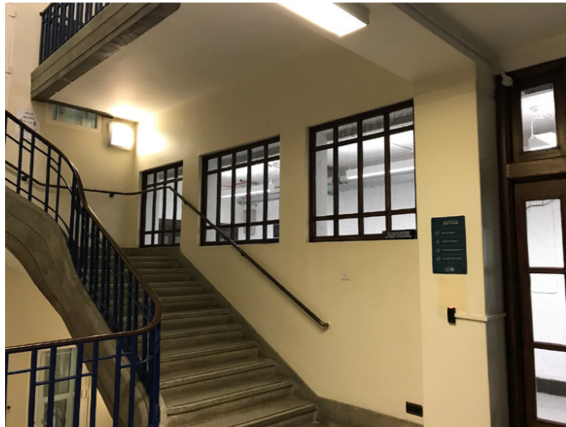
Photograph P5: Stair Core 3 South-West Elevation: Existing Windows at Third Floor (Corridor Side)
