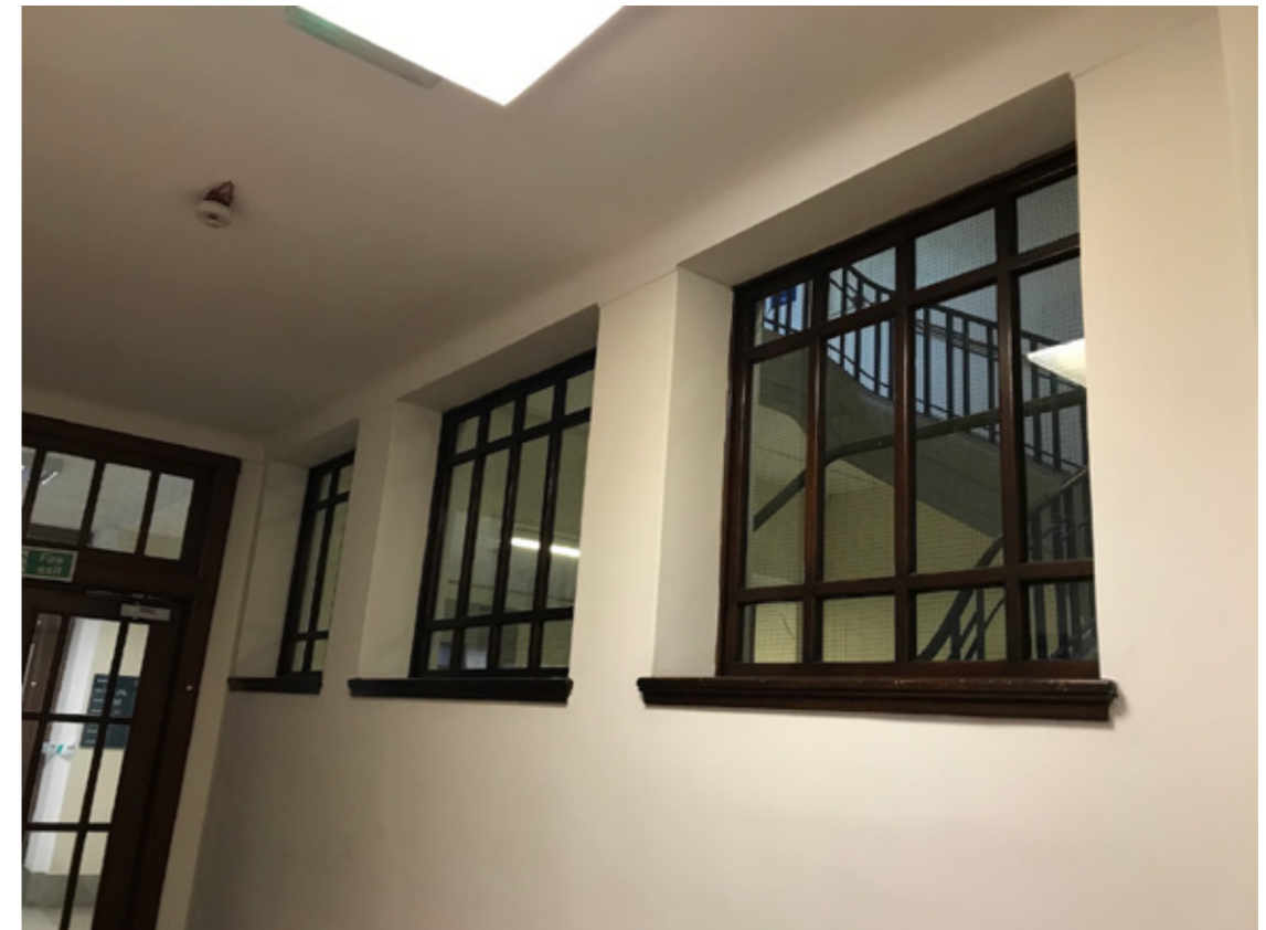
Photograph P8: Stair Core 3 South-West Elevation: Existing Windows at Ground Floor (Corridor Side)
