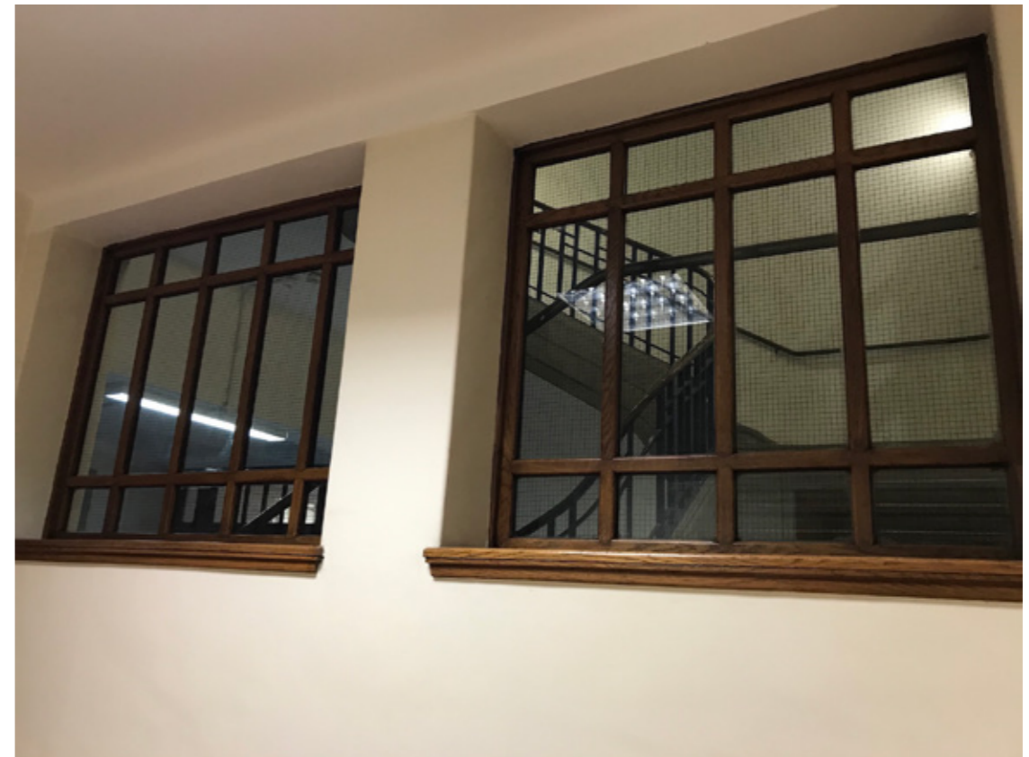
Photograph P7: Stair Core 3 South-West Elevation: Existing Windows at First Floor (Corridor Side)
