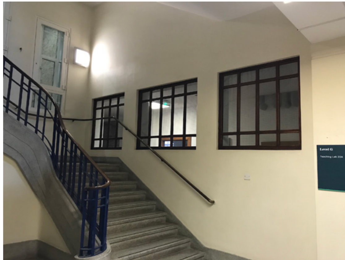
Photograph P7: Stair Core 3 South-West Elevation: Existing Windows at Ground Floor (Stair Core Side)
