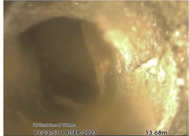
SVPX_5dd9993d-6e49-4d4e-ac08-df64fb90a7a2_20230921_151231_814.jpg, 00:02:42, 13.68 m Attached deposits, encrustation from 12 o'clock to 12 o'clock, 10% cross-sectional area loss, finish
