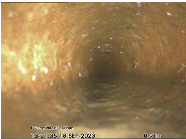
SVPX_deb1f473-a967-4add-ae6d-8fca9d25ea2b_20230921_150847_966.jpg, 00:00:19, 0.56 m Attached deposits, encrustation from 12 o'clock to 12 o'clock, 10% cross-sectional area loss, start
