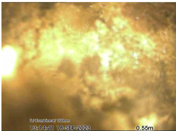
CAPPEDX_08163fef-71cd-44a0-8040-53f6ea637f7be_20230921_150645_318.jpg, 00:00:10, 0.15 m Settled deposits, hard or compacted, 15% cross-sectional area loss
