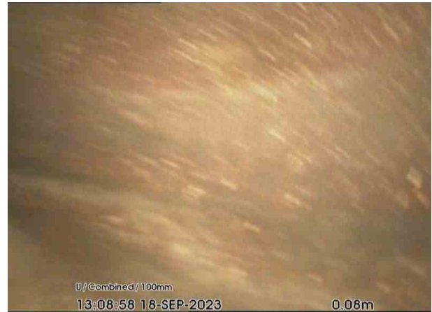
RWGX_12e78270-e1b2-499e-b6f2-51f7e6173fd1_20230921_150428_416.jpg, 00:00:08, 0.05 m Line deviates left
