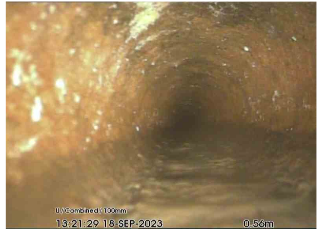
SVPX_eb52a971-7362-471b-afde-9110ca26785b_20230921_150843_929.jpg, 00:00:19, 0.56 m Attached deposits, encrustation from 12 o'clock to 12 o'clock, 10% cross-sectional area loss, start
