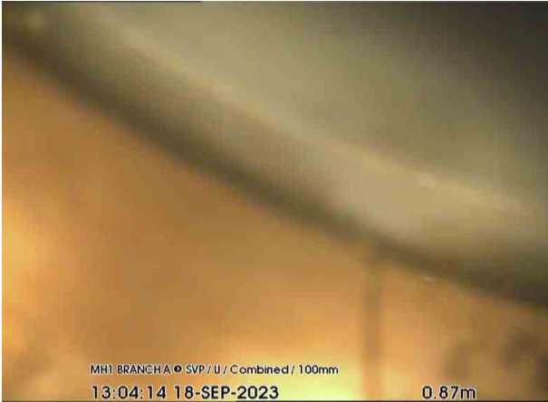
SVPX_70276489-0269-4ed0-8edc-229f7ae8107b_20230921_150217_683.jpg, 00:00:36, 1.27 m Finish node, other special chamber, reference: SVP, REACHED
