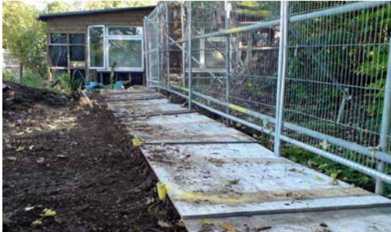
SGN 3-02 Heavy-duty plywood set onto a compressible woodchip layer and pinned into position is suitable to spread the loading from pedestrian access.
