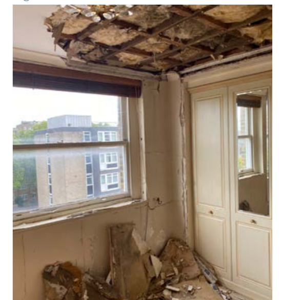
Collapsed ceiling at third floor bedroom
