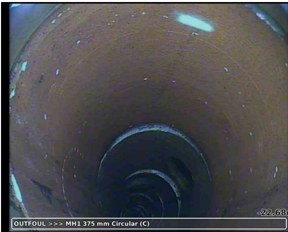
20230927-163711-snap0011.jpg, 00:02:35, -22.68 m Connection defective, position incorrect at 10 o'clock, diameter: 3mm
