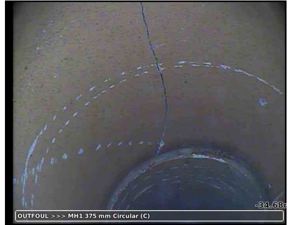
OUTFOUL >>> MH1 375 mm Circular (C) 20230927-163711-snap0020.jpg, 00:03:42, -34.64 m Crack, longitudinal at 12 o'clock, start
