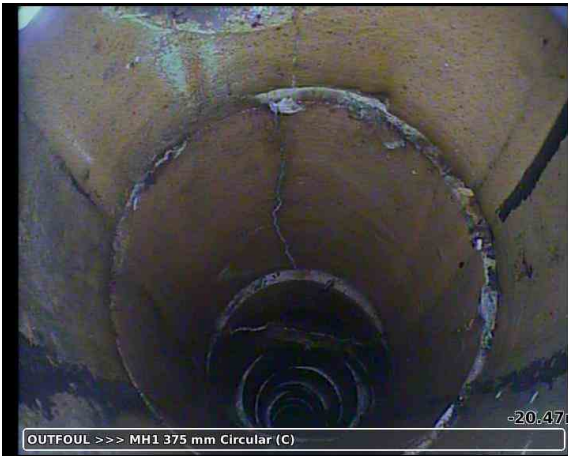
20230927-163711-snap0009.jpg, 00:02:21, -20.47 m Crack, longitudinal at 12 o'clock, start
