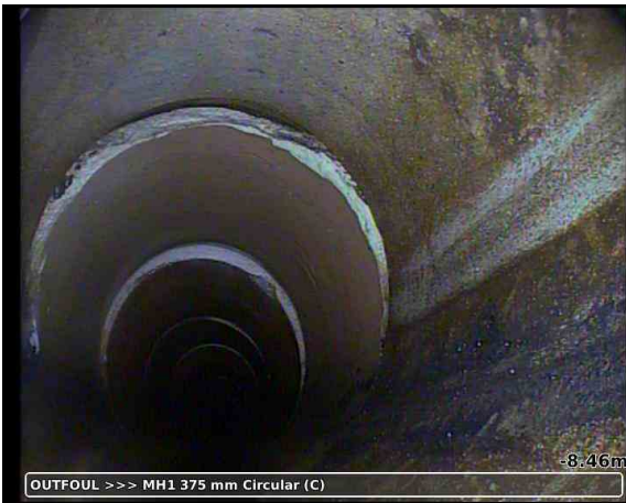
20230927-163711-snap0003.jpg, 00:00:58, -8.46 m Connection defective, position incorrect at 3 o'clock, diameter: 6mm
