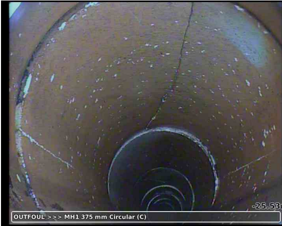
20230927-163711-snap0013.jpg, 00:02:50, -25.53 m Crack, longitudinal at 12 o'clock, start
