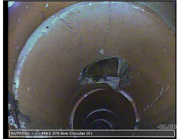
20230927-163711-snap0012.jpg, 00:02:40, -23.28 m Cracks, multiple from 12 o'clock to 4 o'clock, start
