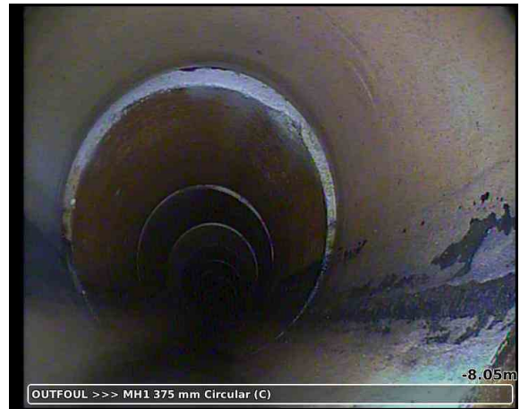
20230927-163711-snap0002.jpg, 00:00:55, -8.05 m Connection defective, position incorrect at 9 o'clock, diameter: 3mm
