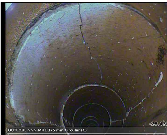
20230927-163711-snap0015.jpg, 00:03:04, -28.43 m Crack, longitudinal at 12 o'clock, start
