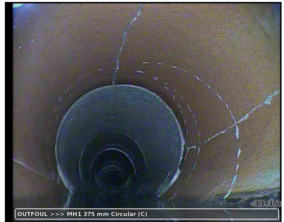
OUTFOUL >>> MH1 375 mm Circular (C) 20230927-163711-snap0018.jpg, 00:03:33, -33.35 m Crack, longitudinal at 12 o'clock, start
