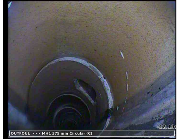
20230927-163711-snap0004.jpg, 00:01:25, -12.19 m Connection defective, position incorrect at 11 o'clock, diameter: 5mm
