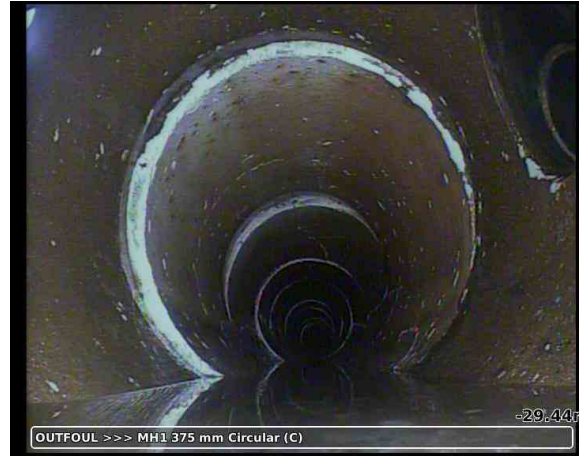
20230927-163711-snap0016.jpg, 00:03:09, -29.44 m Connection defective, position incorrect at 7 o'clock, diameter: 3mm
