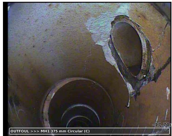
20230927-163711-snap0006.jpg, 00:02:03, -17.76 m Cracks, multiple at joint from 3 o'clock to 6 o'clock, start
