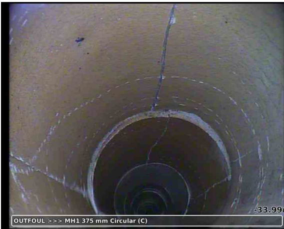
OUTFOUL >>> MH1 375 mm Circular (C) 20230927-163711-snap0019.jpg, 00:03:37, -33.99 m Crack, longitudinal at 12 o'clock, start
