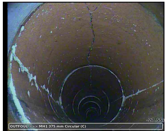
20230927-163711-snap0014.jpg, 00:03:00, -27.55 m Crack, longitudinal at 12 o'clock, start
