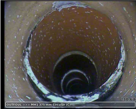
20230927-163711-snap0017.jpg, 00:03:20, -30.64 m Connection defective, position incorrect at 3 o'clock, diameter: 9mm
