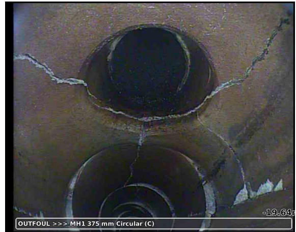
20230927-163711-snap0008.jpg, 00:02:16, -19.64 m Cracks, multiple from 9 o'clock to 4 o'clock, start
