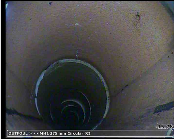
20230927-163711-snap0005.jpg, 00:01:47, -15.78 m Crack, longitudinal at 12 o'clock, start
