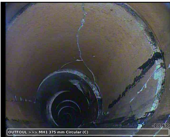
20230927-163711-snap0007.jpg, 00:02:10, -18.68 m Crack, longitudinal at 12 o'clock, start
