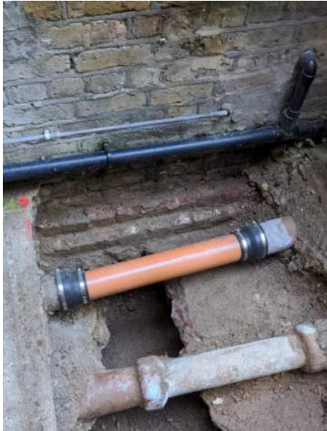
Plate 5. Presence of shallow services at corridor level
