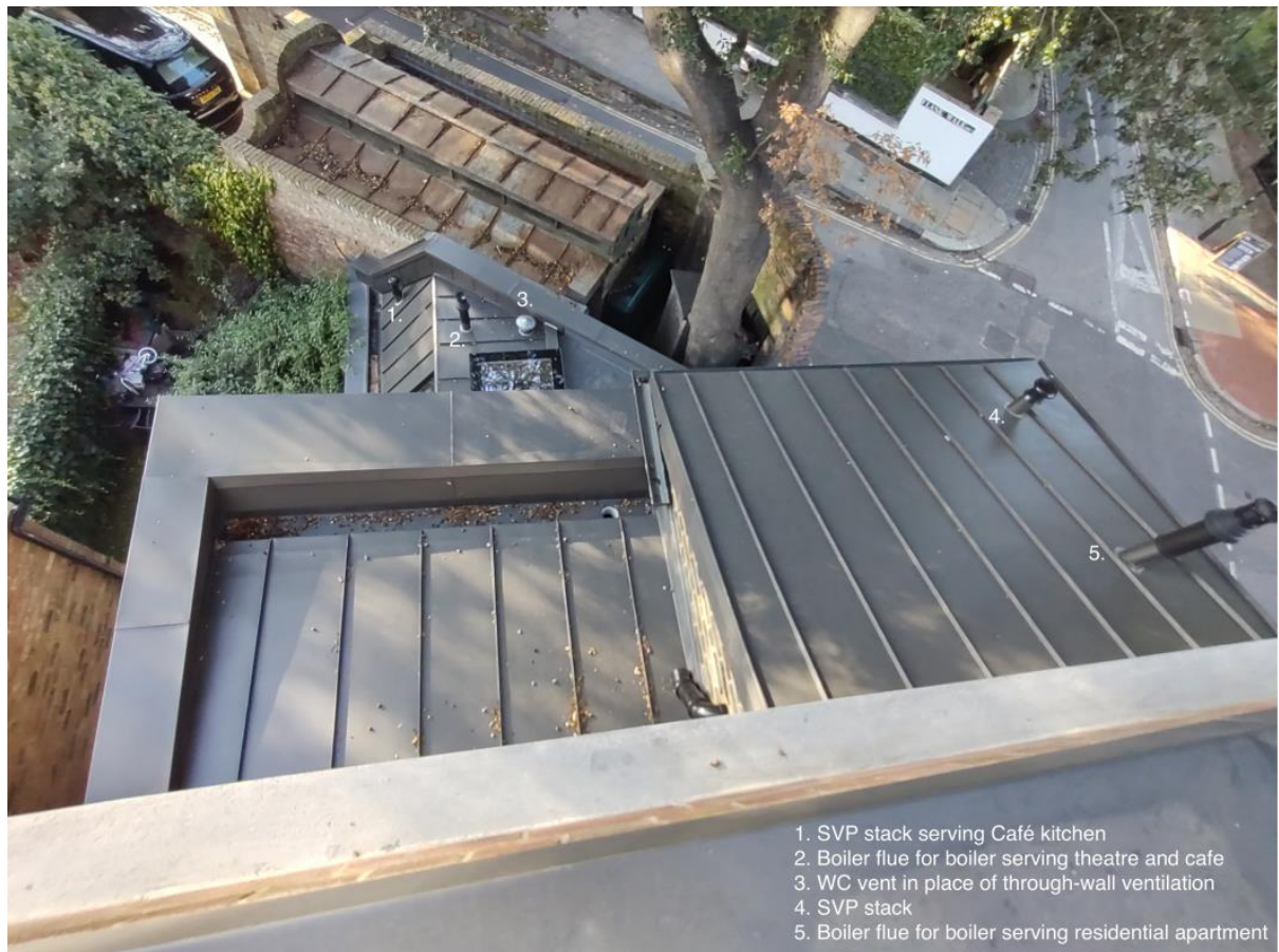
Photo 1: Location of 2 x SVP stacks, 2 x boiler flues and WC vent
