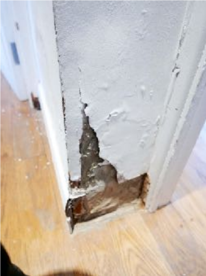
PHOTO 5: Dividing Wall between lounge and kitchen showing damp wall and cracking/peeling fabric.
