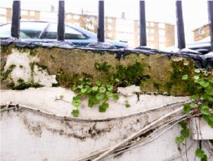
PHOTO 3: Damp retaining wall to the sunken area, resulting in cracked and crumbling fabric.
