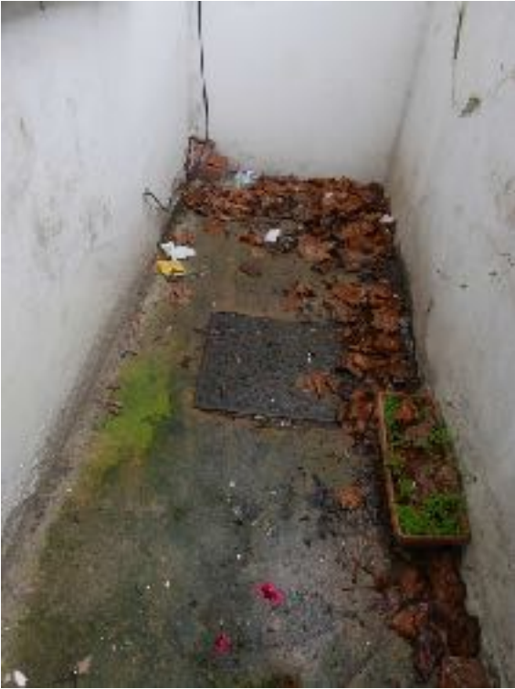
PHOTO 1: Front “Sunken “ area showing the damp in the external wall.
