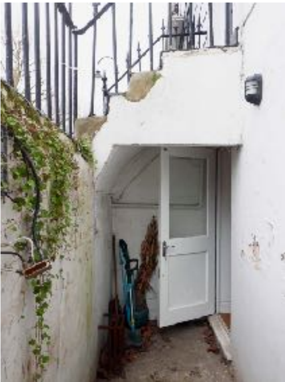
PHOTO 2: Front external area with access door, showing damp wall on the external elevation.
