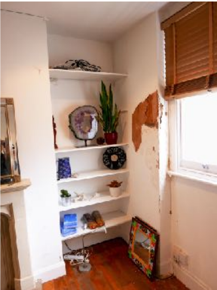
PHOTO 4: Damp and cracking fabric in the "Lounge" area. (External Wall).
