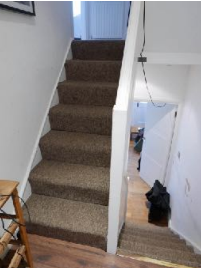
PHOTO 5: Damp and cracking fabric in party wall along the stair from basement to mezzanine level.
