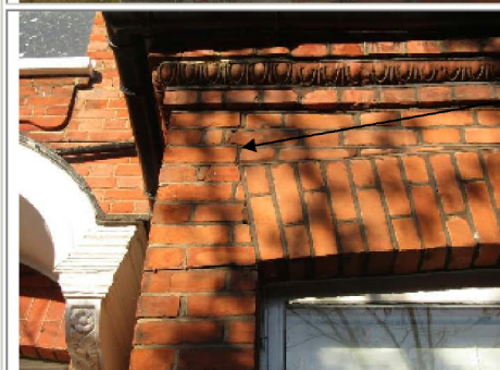
Photograph 6 front RHS bay – above window
