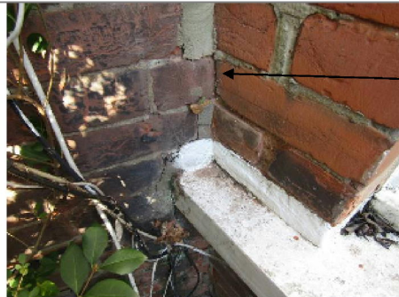
Photograph 10 front LHS bay – below window
