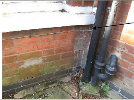
Photograph 8 front LHS bay – below window
