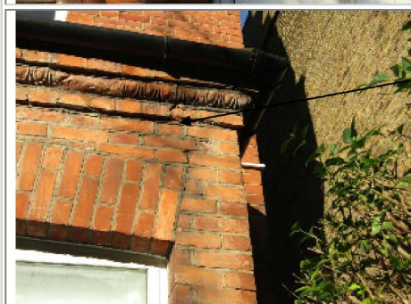
Photograph 7 front RHS bay – above window
