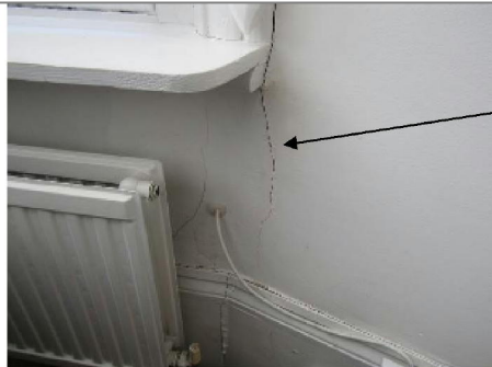
Photograph 14 Front LHS bedroom – below bay window
