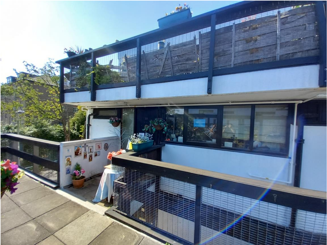
Figure 1 Photograph of the installed pipework at first floor level.
