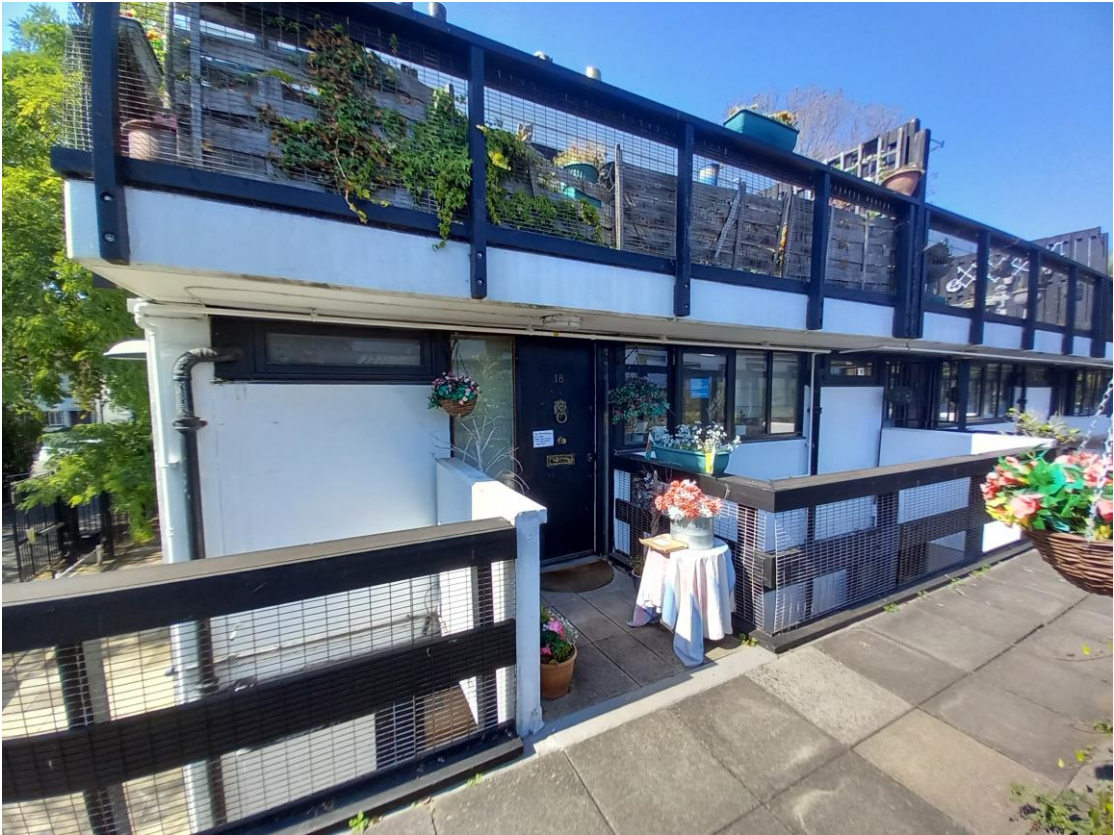
Figure 2 Photograph of the installed pipework at first floor level.
