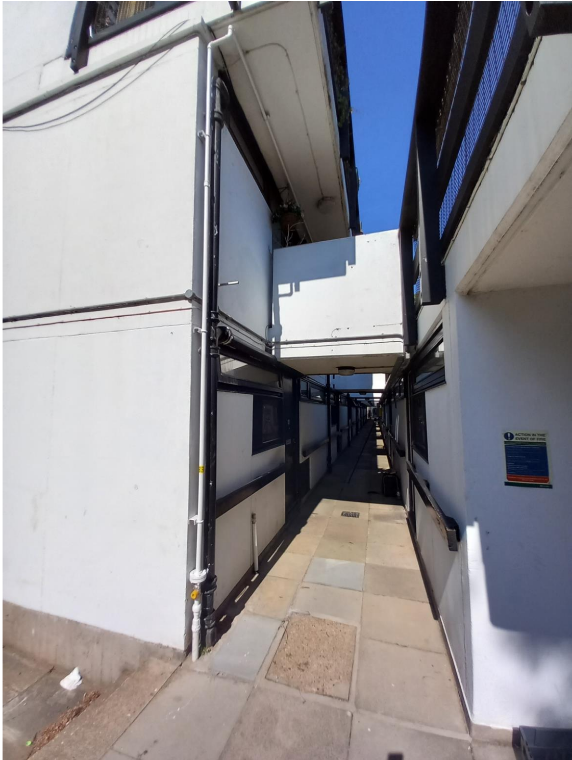
Figure 3 Photograph of the installed pipework at ground and first floor level.
